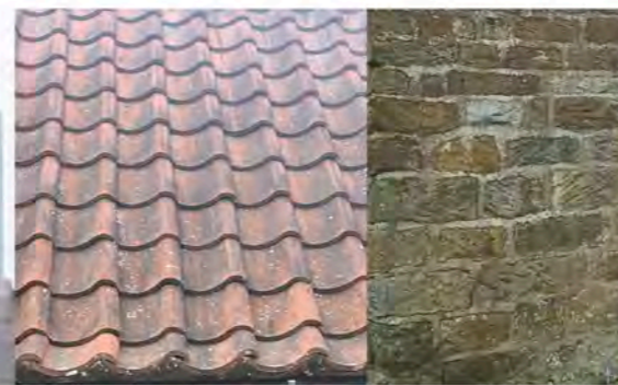
Reuse of clay pantiles, where practical, on the new roof to the main house Stone walls to the main house to be re-pointed
