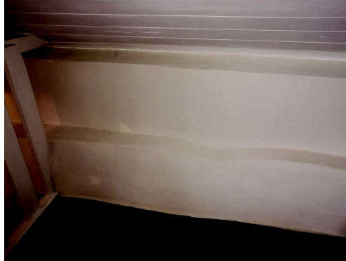
Fig 5 - Stepped internal southern wall showing differing thickness of brick and stone courses
