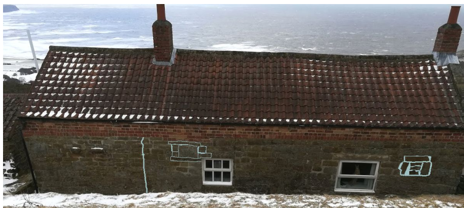
Fig 4 - Southern elevation showing likely filled apertures, break in building line and insertion of bricks at eaves level
