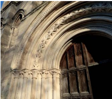
Hot applied sheltercoat to protect eroding sculpture at St Mary's Church, Old Malton
