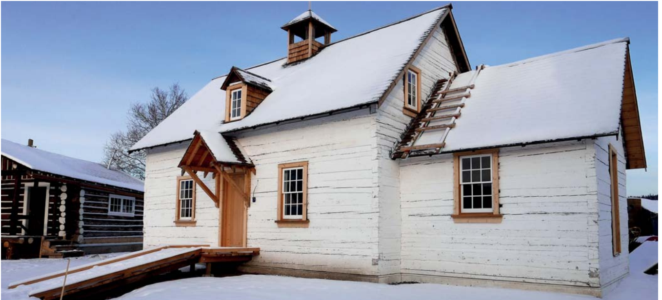
Hot limewash with salt on the timber walls of the French Jesuit Mission Church (1910) at Fort McMurray, Alberta (Photo: Ben Gourley, MacDonald and Lawrence Timber Framers)
