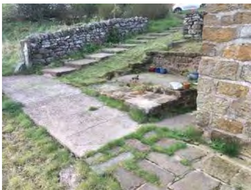
Fig 5. – shows concrete steps, concrete foundation and pad to side of property (north and east)
