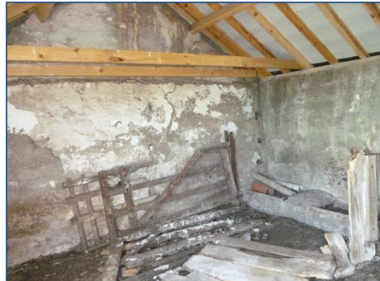
Photo 5: Interior with barn owl pellets and streaking
