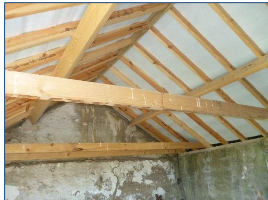
Photo 7: Internal roof structure and bird droppings on beam.
