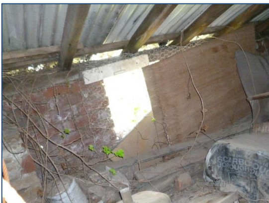
Photo 6: Section B gaps under corrugated roof and mesh over window.
