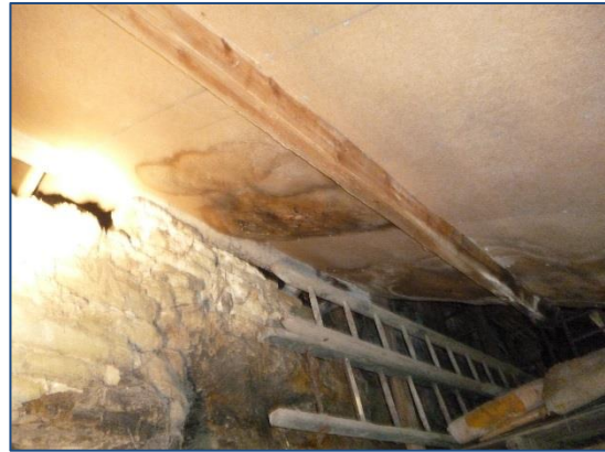
Photo 3: Section A roof boarding with damp.
