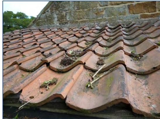
Photo 11: Loose tiles on lean-to rood of rooms C and D.
