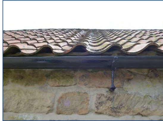
Photo 3: Gaps under eaves.
