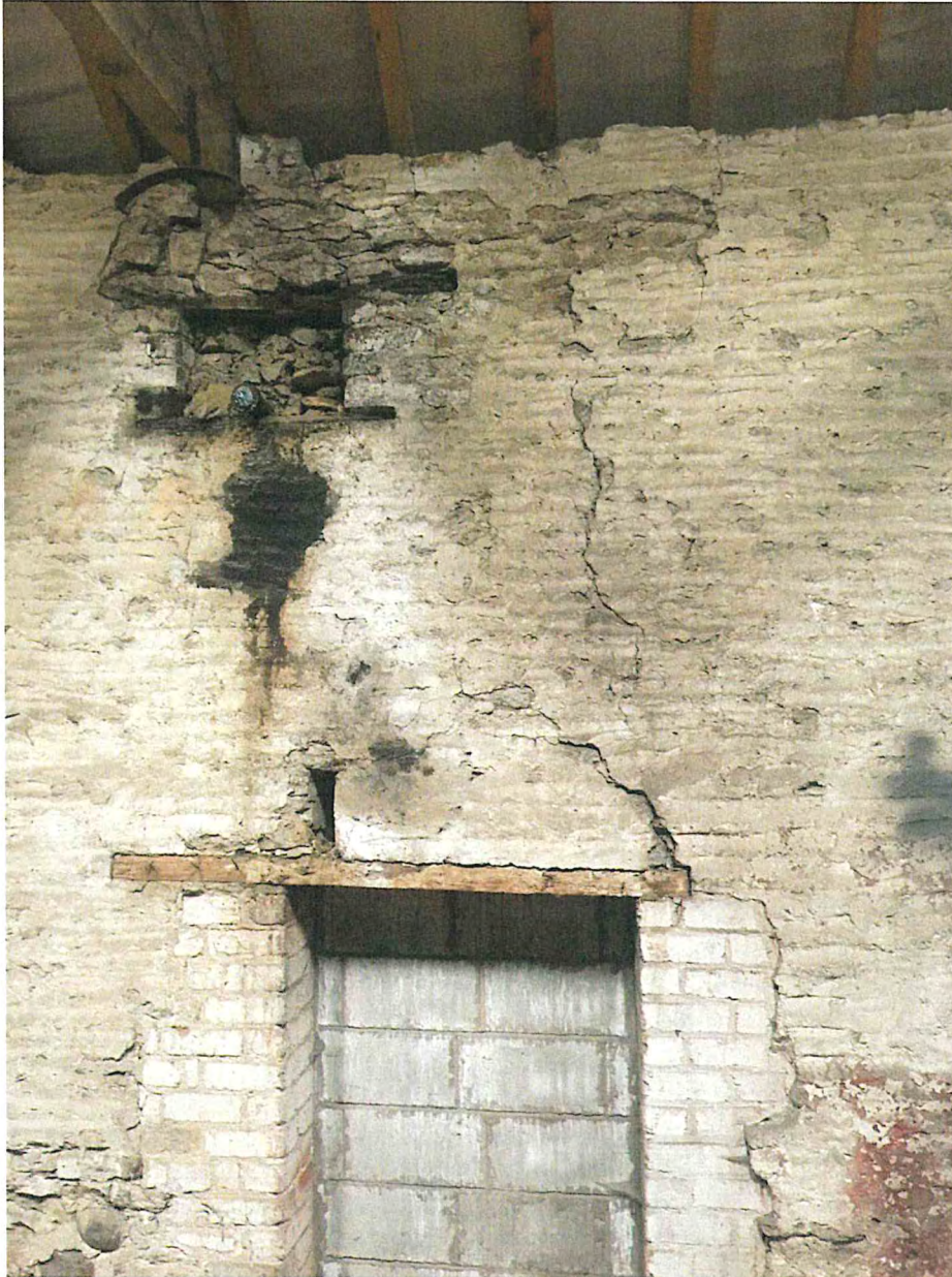
Photograph 13 – cracking in wall below roof truss
