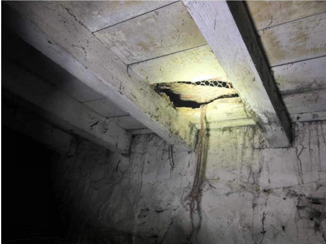
Image 7. Hole in ceiling of storage room.
