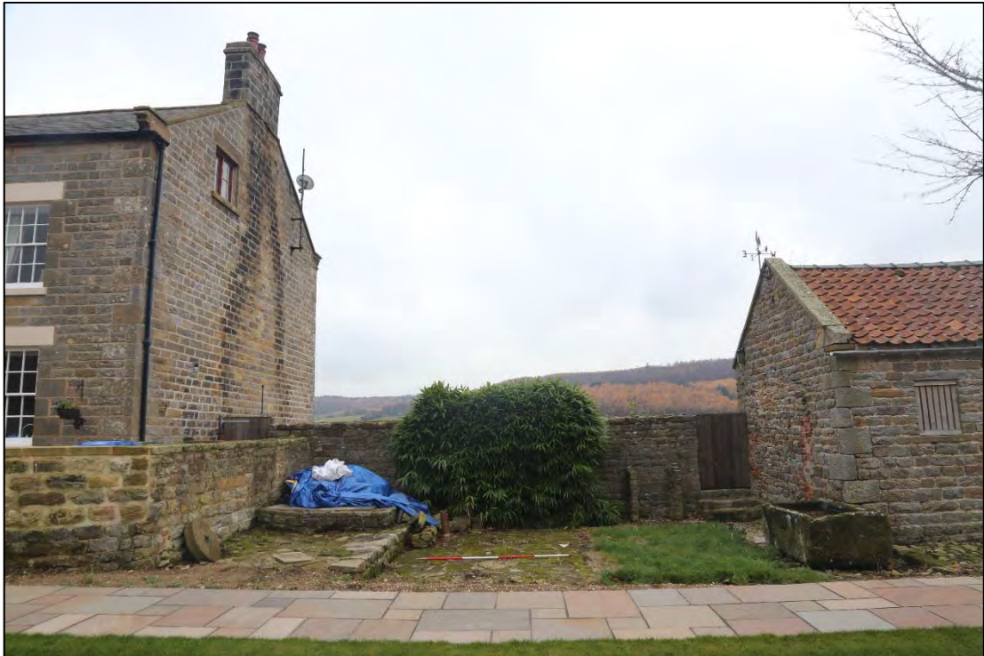
Plate 61: building footings between the south range and farmhouse associated with the south range extension. This building may have originally served as an implement shed or pigsty.
