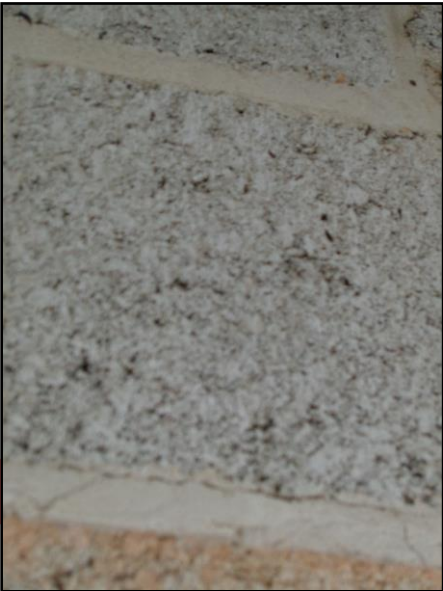
Figure 37. Bat droppings across walls in the corner of south eastern barn below possible roost entrance
