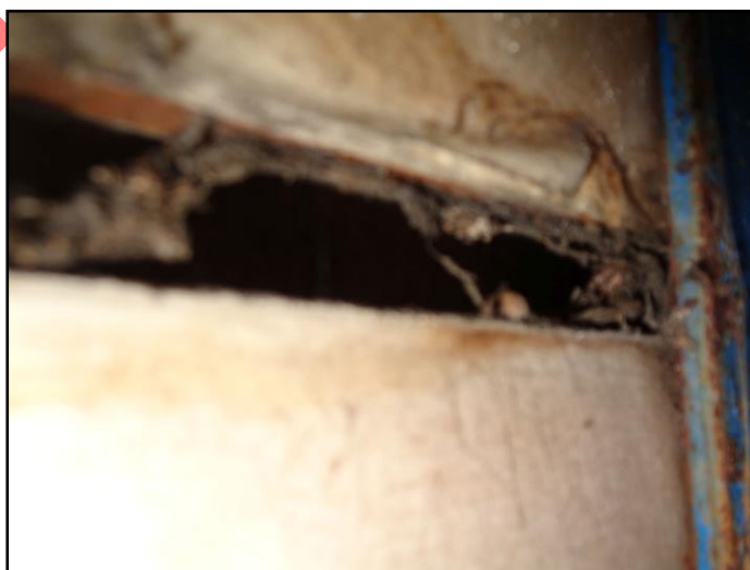
Figure 27. First floor – some area heavily cobwebbed
