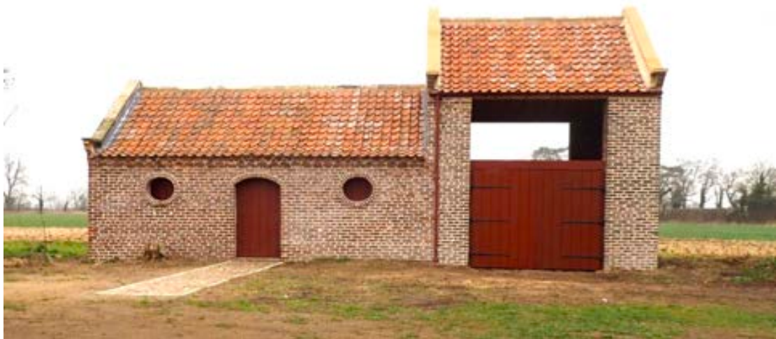
Nawton Towers, Pockley. 1 year after repointing:
