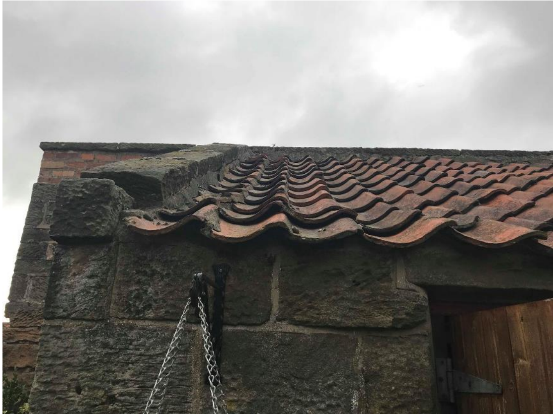
Image 2. South elevation of roof showing gaps under tiles
