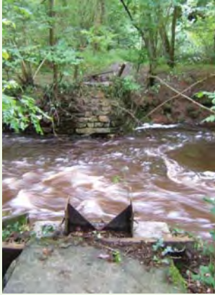
Flood Damage at May Beck
