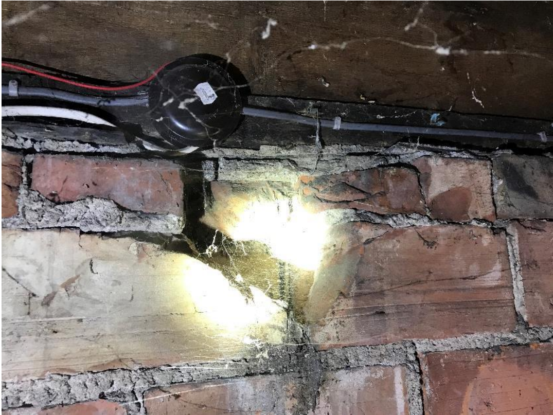
Image 8. Example of heavy cobwebbing in utility area.
