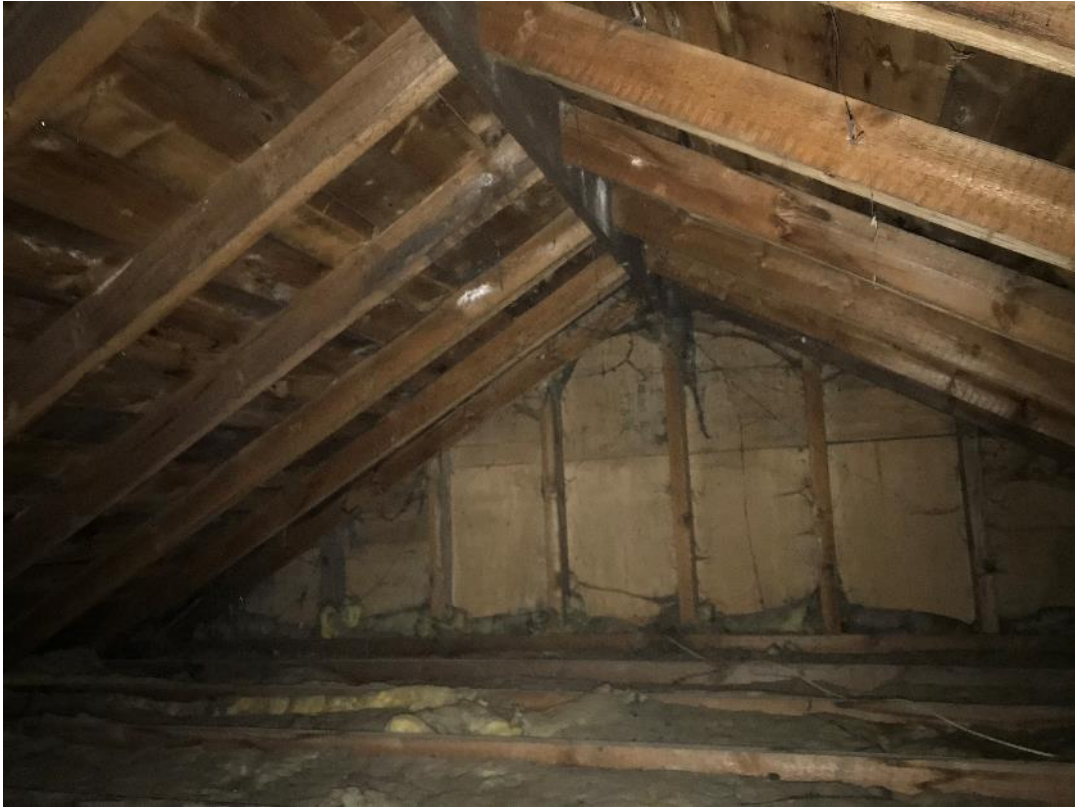
Image 6. One of the roof spaces of the main property, with heavy cobwebbing.
