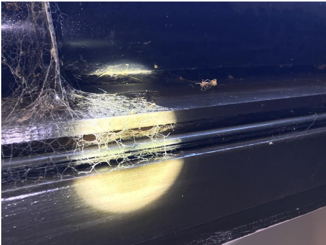
Image 3. Gap behind fascia on porch, with cobwebs and detritus.
