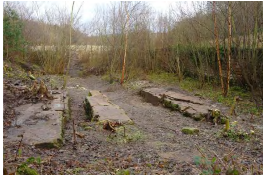
Remnant stone block foundations at Grinkle Mine, scrub encroachment to be managed and interpretation panel provided.
