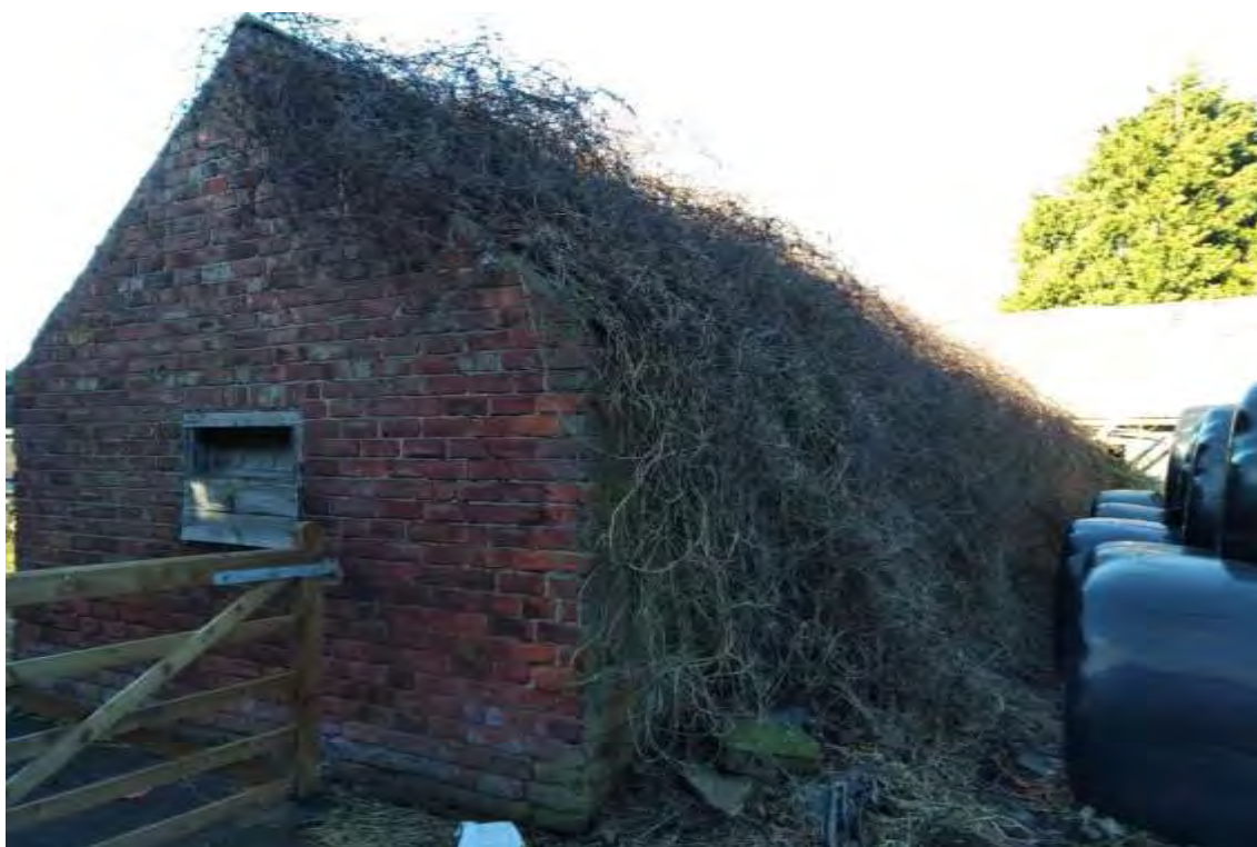
Photograph 5 Building 4, eastern and southern aspect. Roof in poor condition and damaged due to climbing plant.
