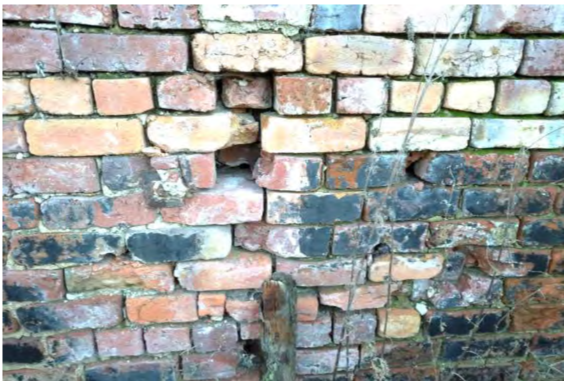
Photograph 13 Brick wall between buildings 8 & 9 showing deep cracks in brickwork, some of which lead deep into the cavity.
