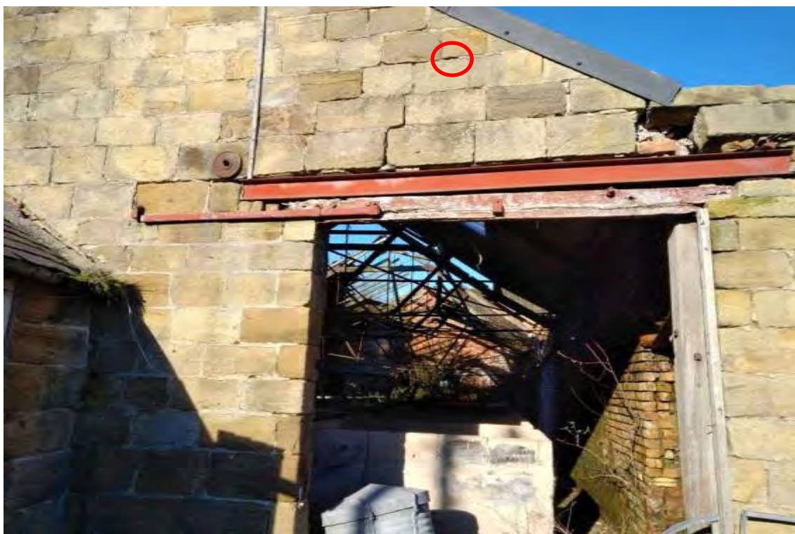
Photograph 17 Cracks in stonework on southern aspect of piggery evident, with former roost site still present (circled) along with larger holes and cracks.
