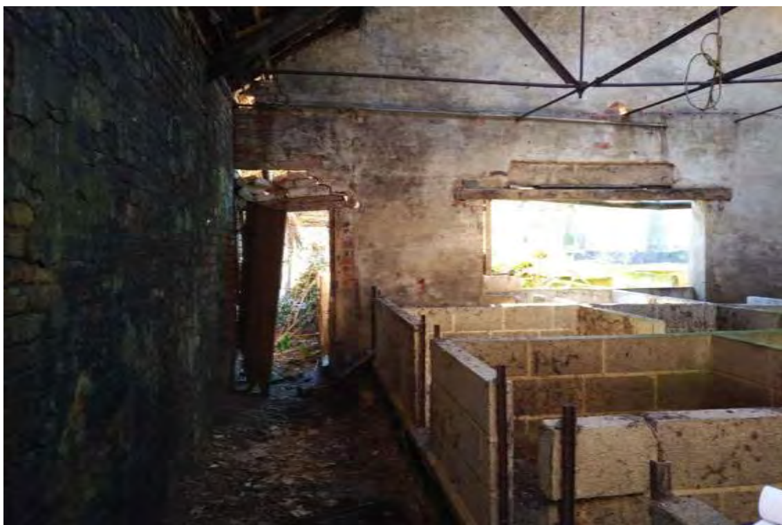
Photograph 15 Northern part of piggery (Building 10) in a state of disrepair, but roof is still standing.
