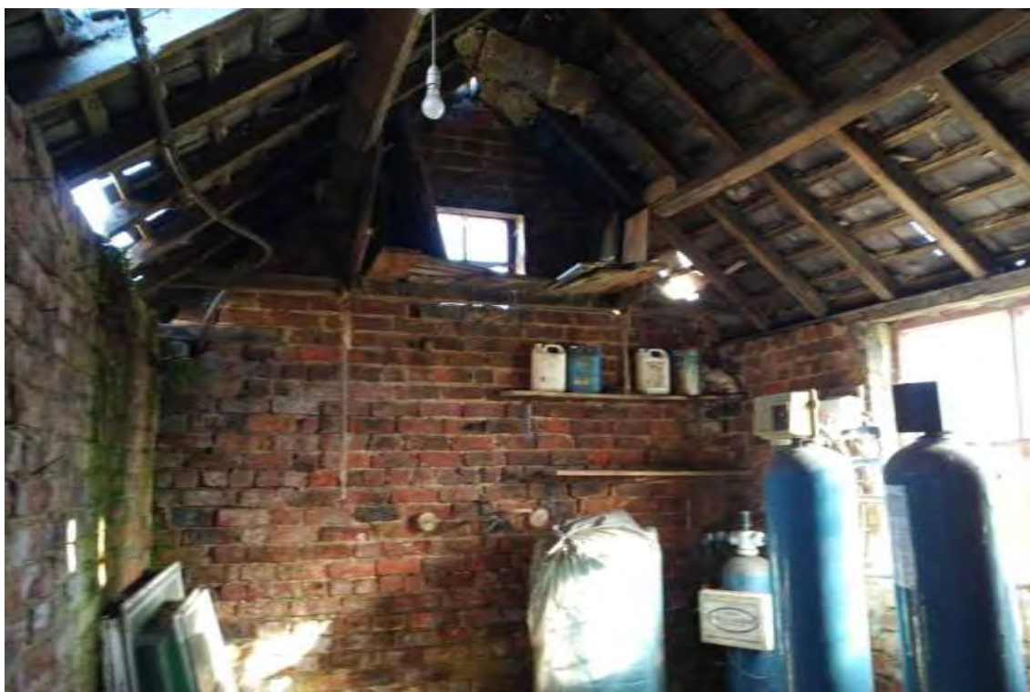
Photograph 19 Building 12 has lots of ridge tiles missing and missing slates. Ridge draughty, negligible potential.
