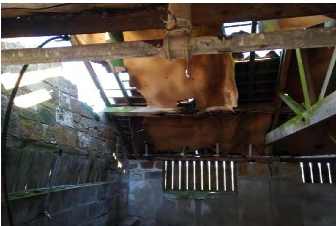
Photograph 12 Building 7, internal structure showing area of missing roof slates at northern end of the building. Building is in a state of disrepair.
