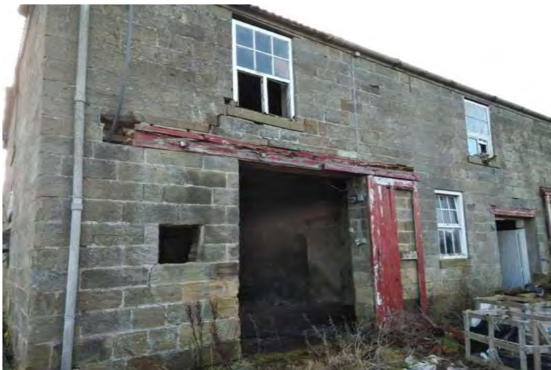
Photograph 9 Building 6, northern aspect showing cracks in stonework due to failing wooden lintel and missing stones.
