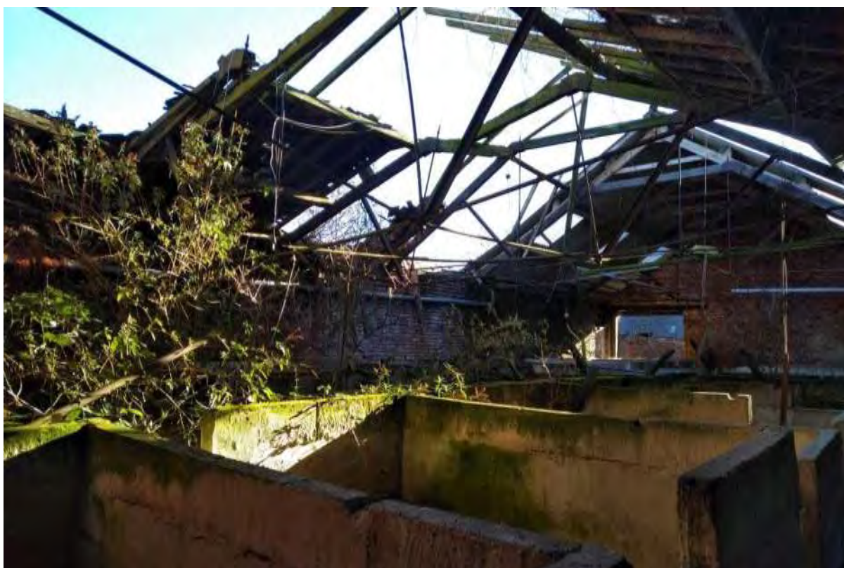
Photograph 16 Southern part of piggery, roof has collapsed exposing it to the elements.
