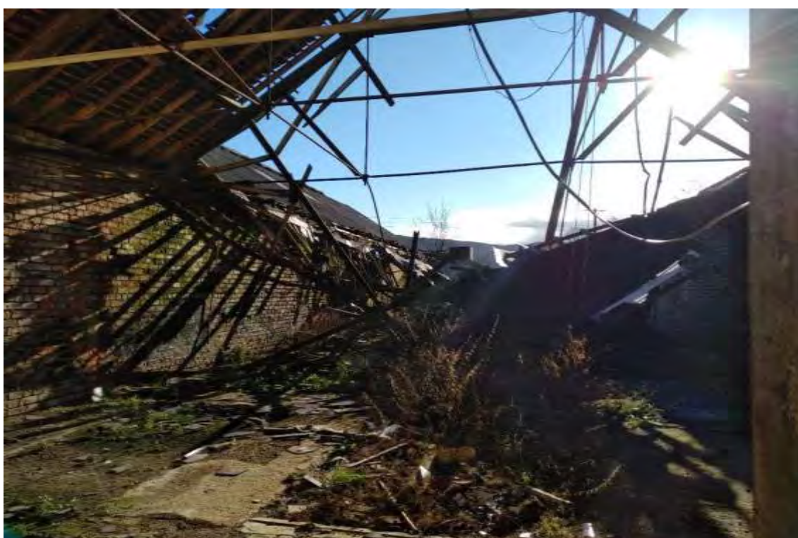
Photograph 14 Building 9 – Roof has collapsed exposing the interior to the elements. Walls with gaps in brickwork remain.
