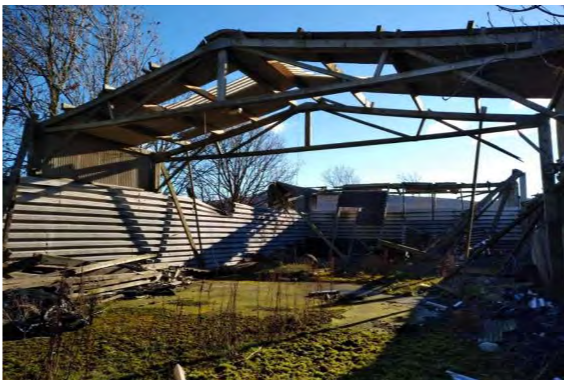
Photograph 20 Building 13, mostly collapsed, just a small central section of roof and corrugated sheet walls remaining.
