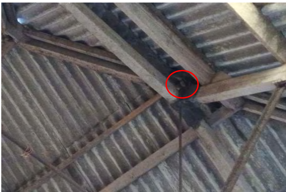
Photograph 10 Building 6, internal roof structure examined through holes in floor. Circled area shows location of roosting tawny owl.
