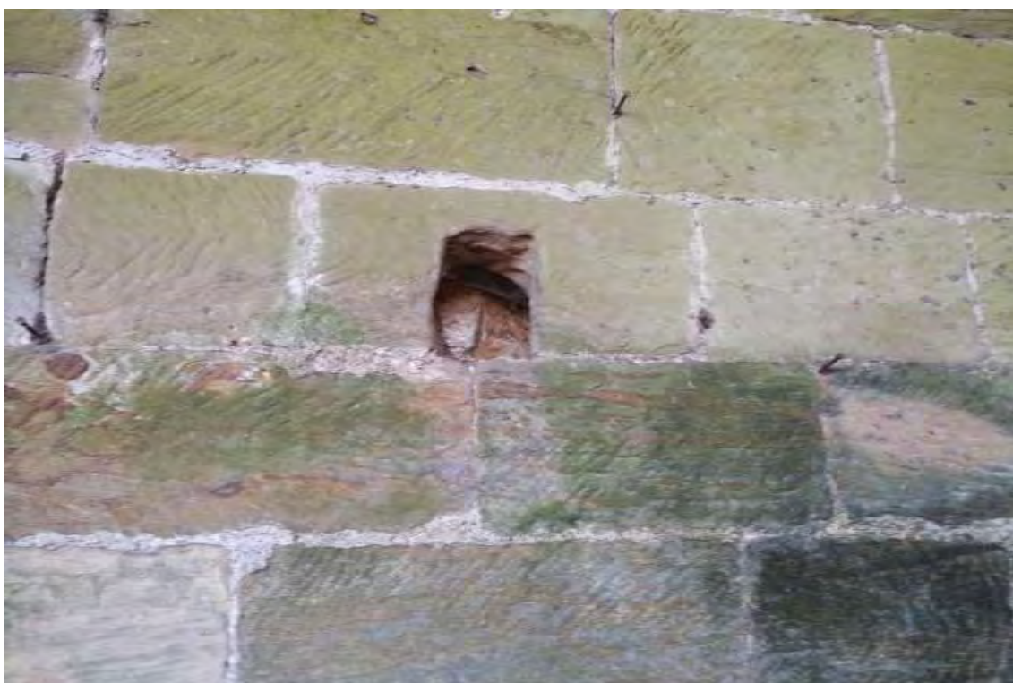
Photograph 8 Interior wall of building 5 showing example of hole in brickwork.
