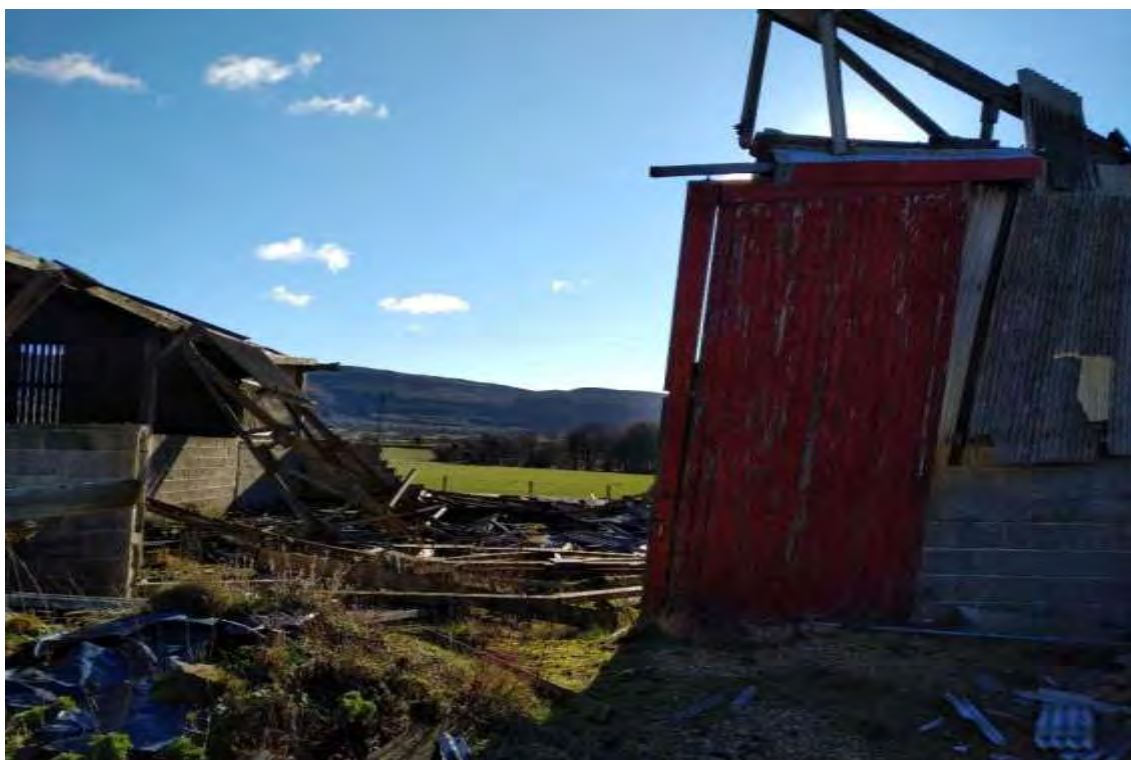
Photograph 21 Western part of Building 14, mostly collapsed.
