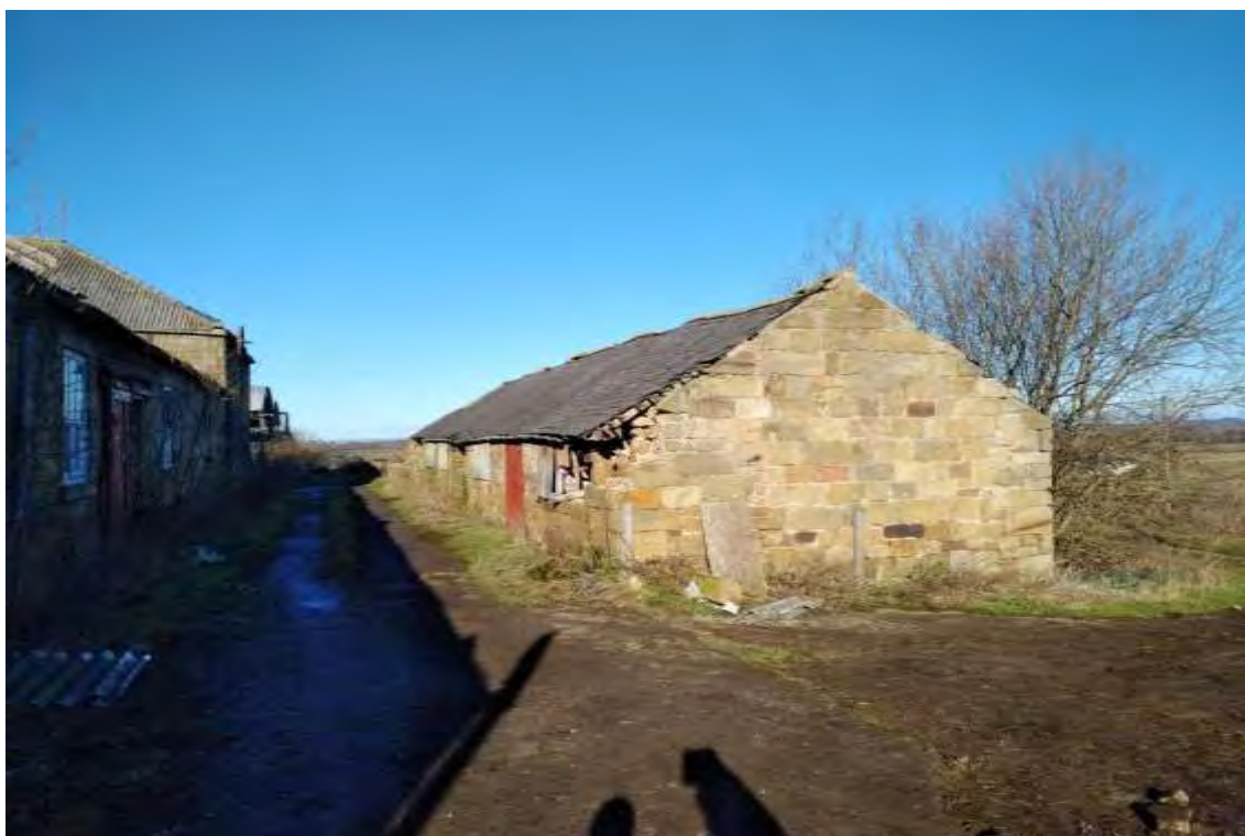
Photograph 11 Building 7, southern and western aspect showing collapsed corner of building.
