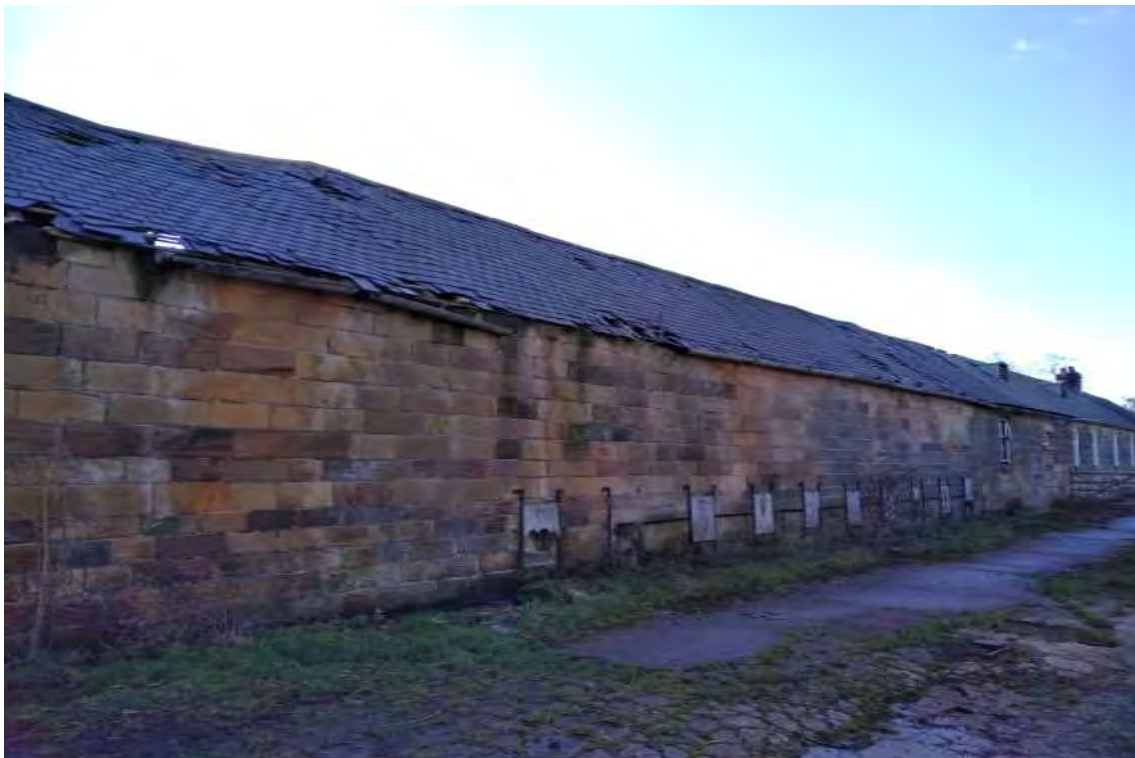
Photograph 4 Building 3 northern aspect. Showing roof in poor condition.
