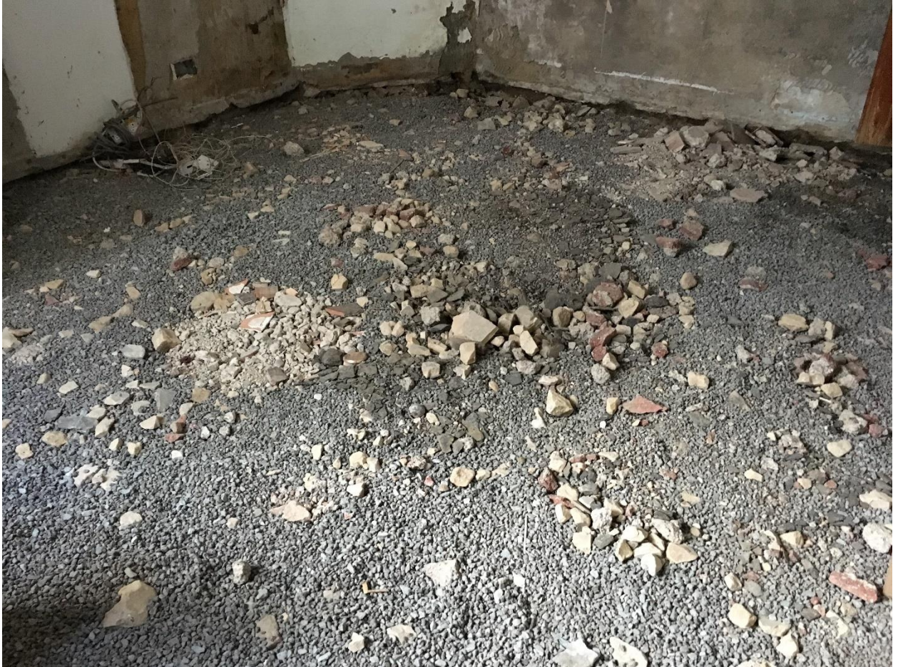
Photograph 1 Kitchen Floor, concrete finish removed, modern inappropriate hardcore exposed
