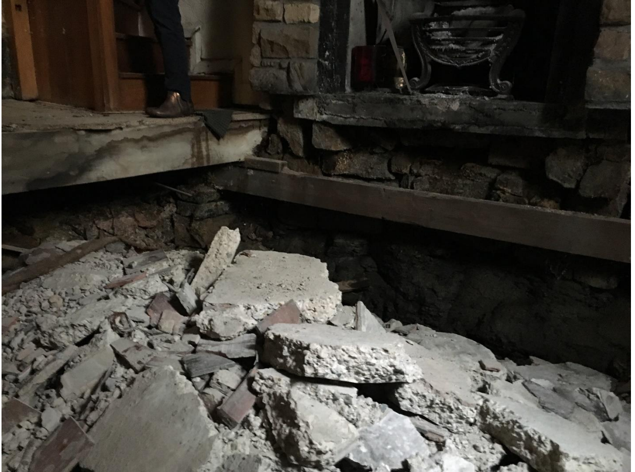
Photograph 4 Lounge floor, void below former timber floor, dumped waste from kitchen floor to be removed
