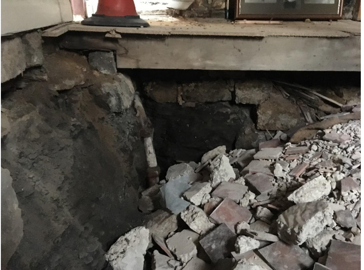
Photograph 3 Lounge floor, void below former timber floor
