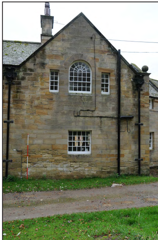
Photograph: 10 Digital Reference: EMBR_033 Description: Detail of one of the gables in the north east elevation of the garages Direction: SW
