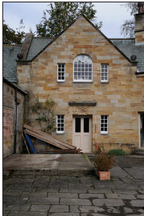
Photograph: 4 Digital Reference: EMBR_025 Description: Gabled South elevation over the keeper's shoot room Direction: N
