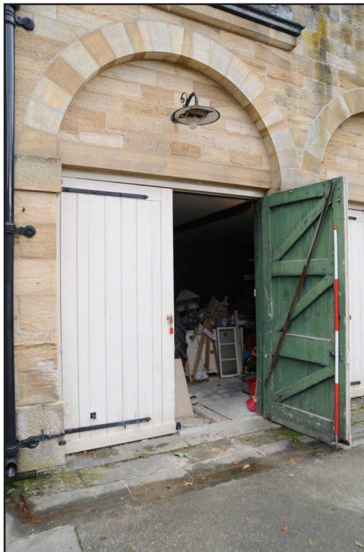
Photograph: 6 Digital Reference: EMBR_029 Description: Semi-circular arch opening into one of the garages Direction: NE
