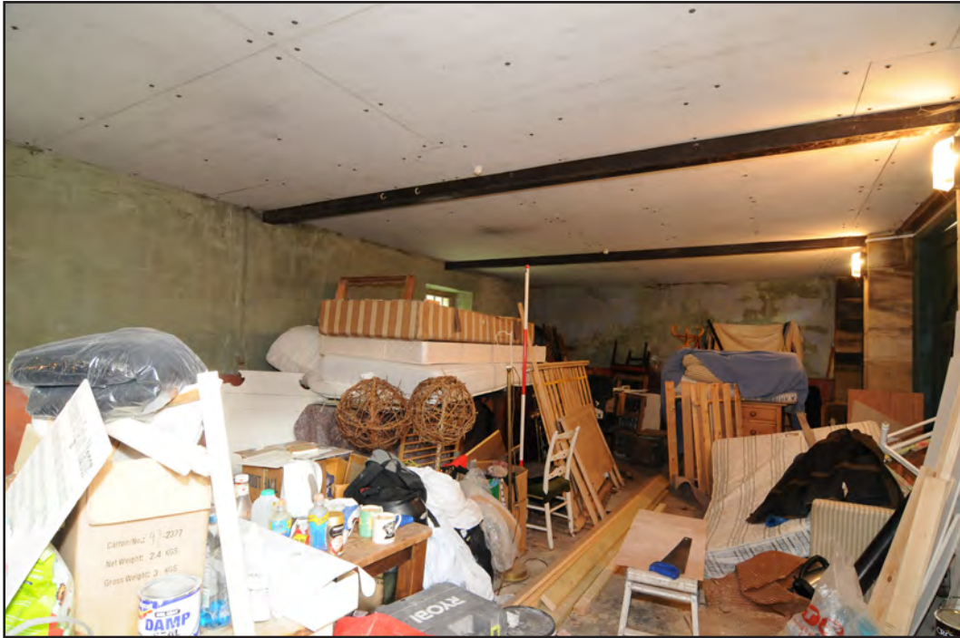
Photograph: 21 Digital Reference: EMBR_068 Description: View inside the garage showing modern plasterboard on the ceiling Direction: E
