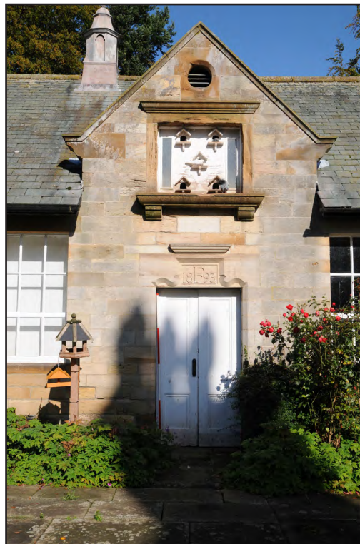
Photograph: 12 Digital Reference: EMBR_019 Description: Gabled entrance porch with the light holes to the dovecote above Direction: N
