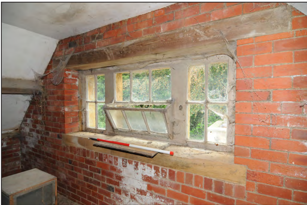
Photograph: 48 Digital Reference: EMBR_064 Description: Detail of the window in the west gable Direction: SW
