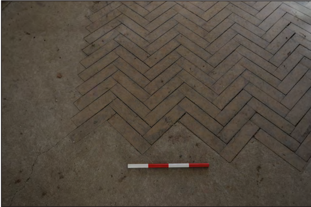
Photograph: 27 Digital Reference: EMBR_010 Description: Remains of the parquet floor surface in the Keepers shoot room Direction: S
