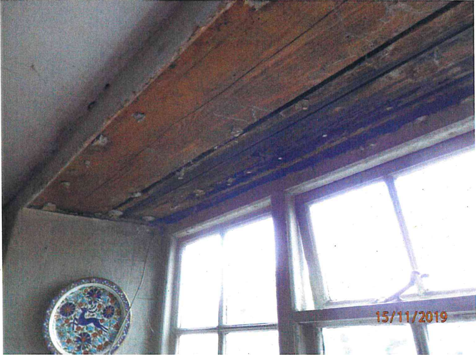
Internal finish to be repaired
