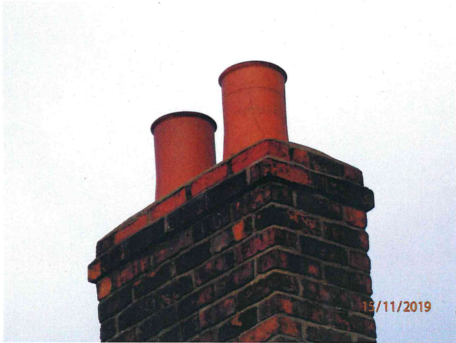
Left Hand side Stack
