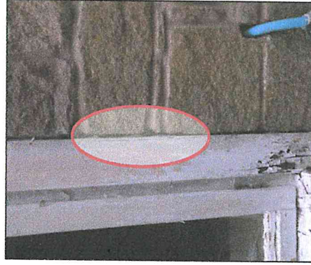
Photo 2. Emergence location at side of window.
