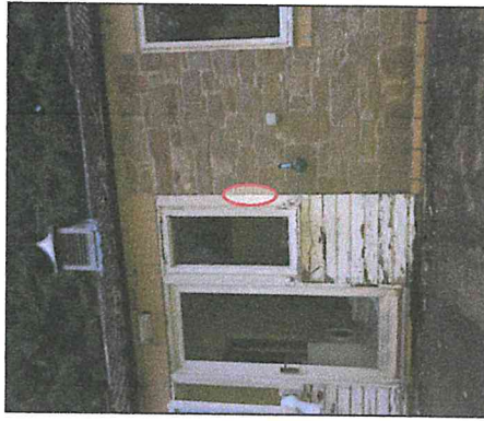
Photo 2. Emergence location at side of window.
