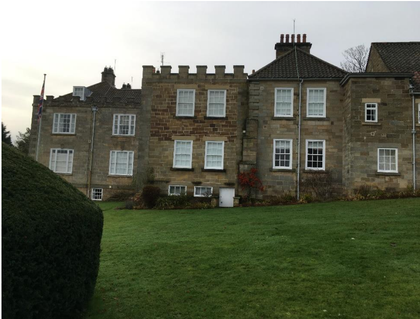
Fig 1. – East elevation with three storey parapet extension (Apartment 11) at The Woodlands, Sleights
