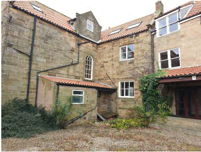
Figure 10: Rear elevation - original building with 1980's extension joining looking North West - Source: Author
