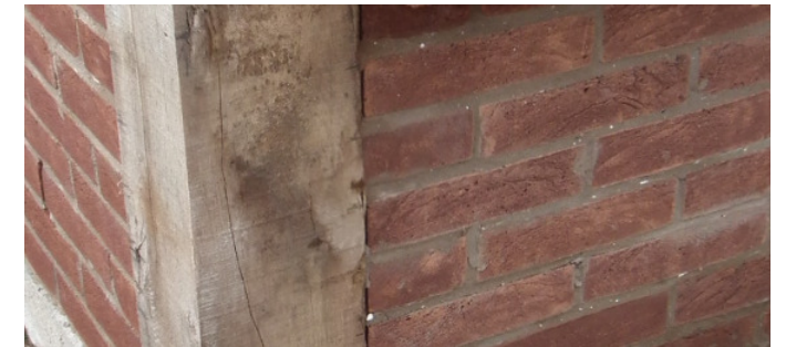
example of oak corner post with specialist brick dwarf wall on brickwork to match the existing dwelling
