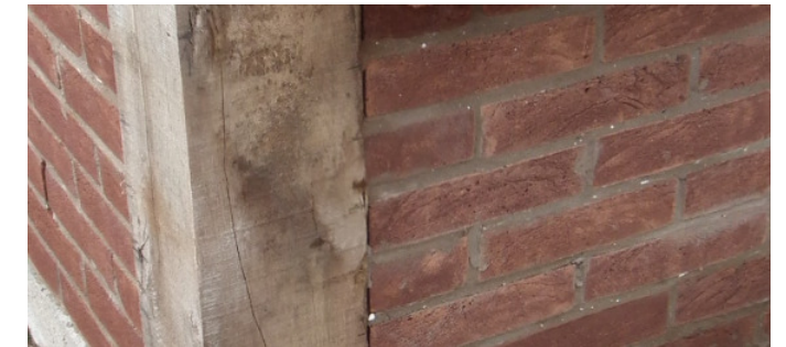
example of oak corner post with specialist brick dwarf wall on brickwork to match the existing dwelling
