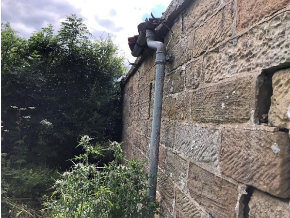
Plate 13 Cracks on exterior walls of Building 2
