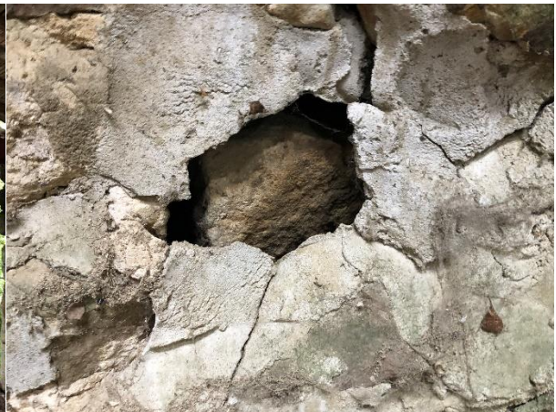
Plate 28 Cracks in interior walls of Building 6
