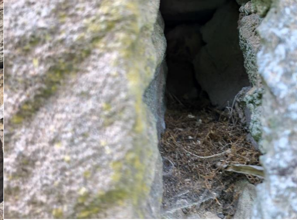
Plate 14 Bird nest within cracks on Building 2
