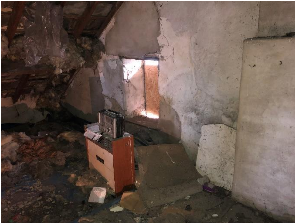
Plate 7 Attic of Building 1 with boarded up window
