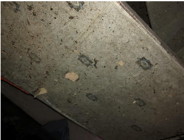
Plate 9 Bat droppings on interior surfaces
