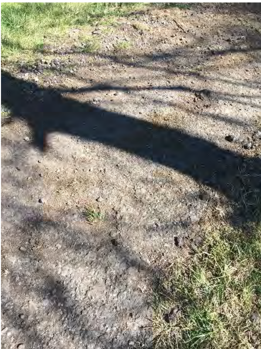
Fig 11. – Identifies tarmac on the bank laid 20 yrs ago. Proof in accounts at Appendix I an J.
