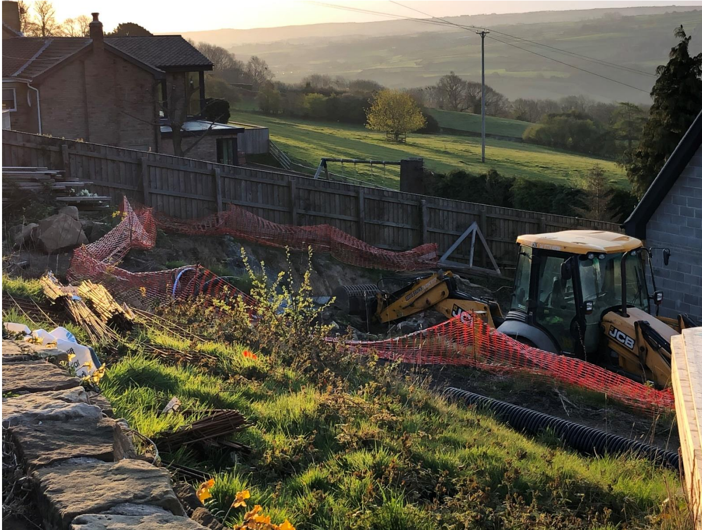
Example 3 - No 21 Significant extensions to dwelling and detached double garage built into rising land. Photo from rear facing Egton Road.
