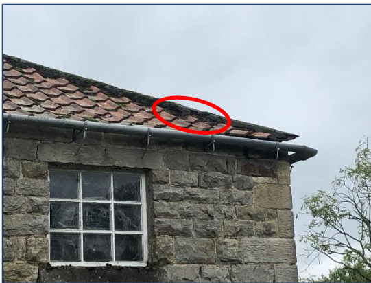
Photo 3: Missing mortar at ridge on Building 1
