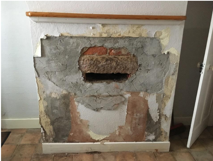
Fig 21. – Ground floor kitchen fireplace with damage walls
