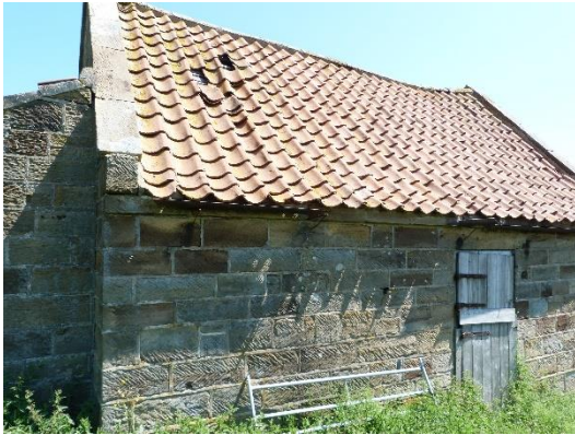
Photo 1 Barn 1 showing missing tiles
