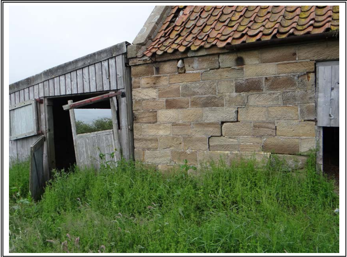
Photo 8 East elevation of Barn B. Note cracking to wall where structural improvements recommended to the intermediate floor and roof structure after a section is rebuilt.
