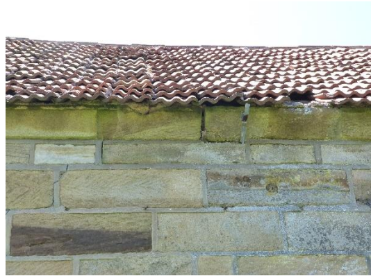
Photo 10 Gaps at eaves in Barn 2
