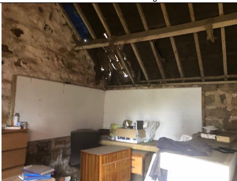
Photograph 28. Showing the storage room/ office with roof damage. Materials in this room provided excellent surfaces to detect droppings, but none were found
