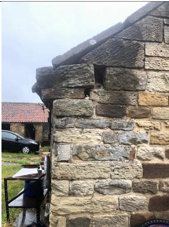
Photograph 5. Showing the coping damage on the south eastern elevation, left hand side.
