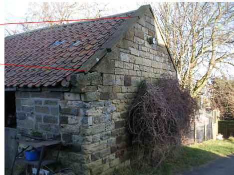
Photograph C loose copings and impact damage
