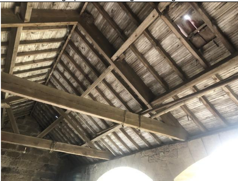
Photograph 20. Showing a view of the timber framework and tile backing of the storage area. Some daylight visible through the roof indicating the damage present
