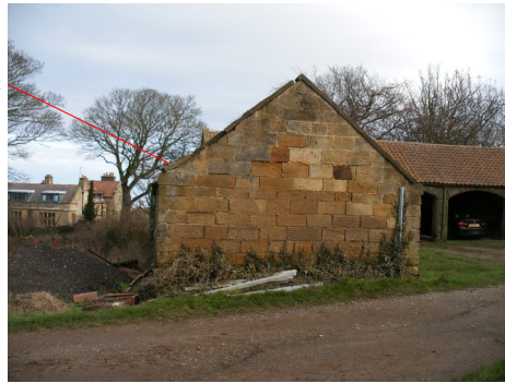
Photograph B impact damage
