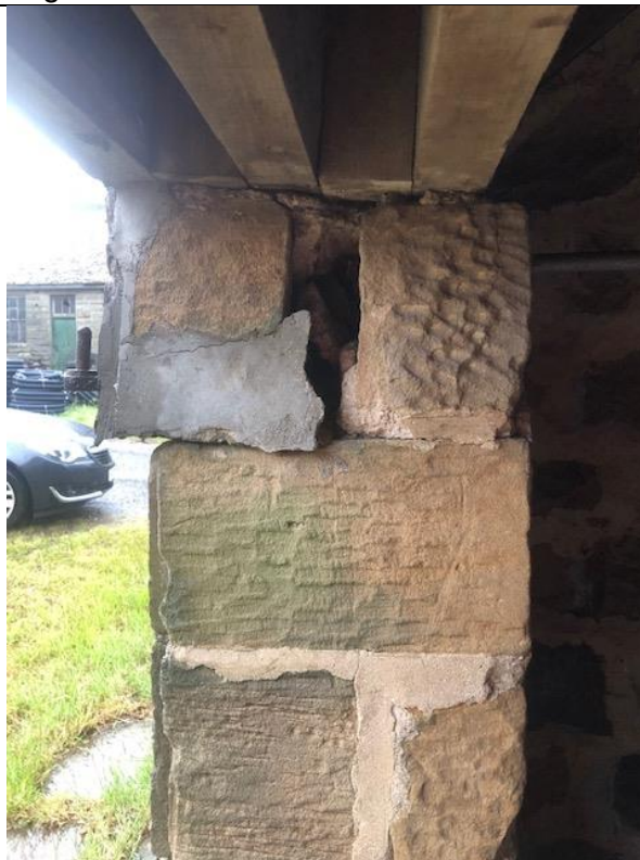
Photograph 26. Showing the gap present in the doorway below the wooden lintel.
