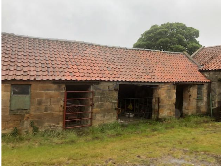
Photograph 1. Showing the external view of the south eastern elevation, including the metal gates, windows present and the damaged roof tiles on the adjoining elevation (on the far right of the picture).
