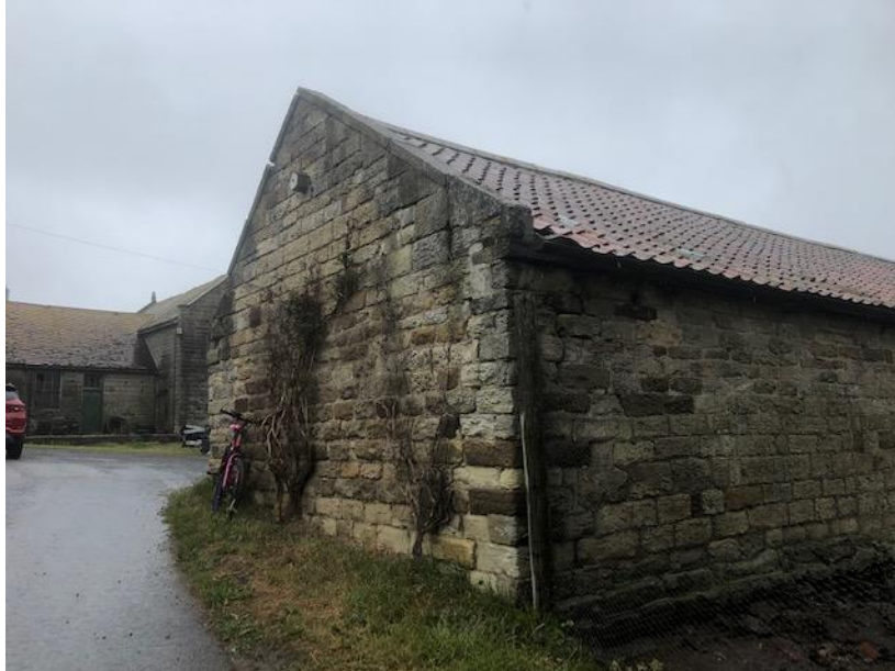
Photograph 4. Showing the external view of the south eastern elevation adjacent to the entrance road, with damage to both sides and coping stones
