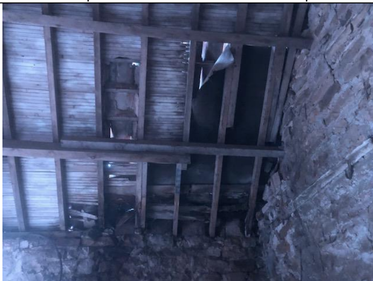
Photograph 22. Showing the roof damage at the gable wall and some more detail of the roof structure (felt present).
