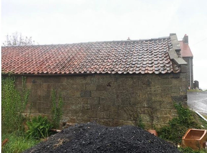
Photograph 13. Showing the end of the north western elevation with damage to the coping stones and roof tiles to the right of the picture.
