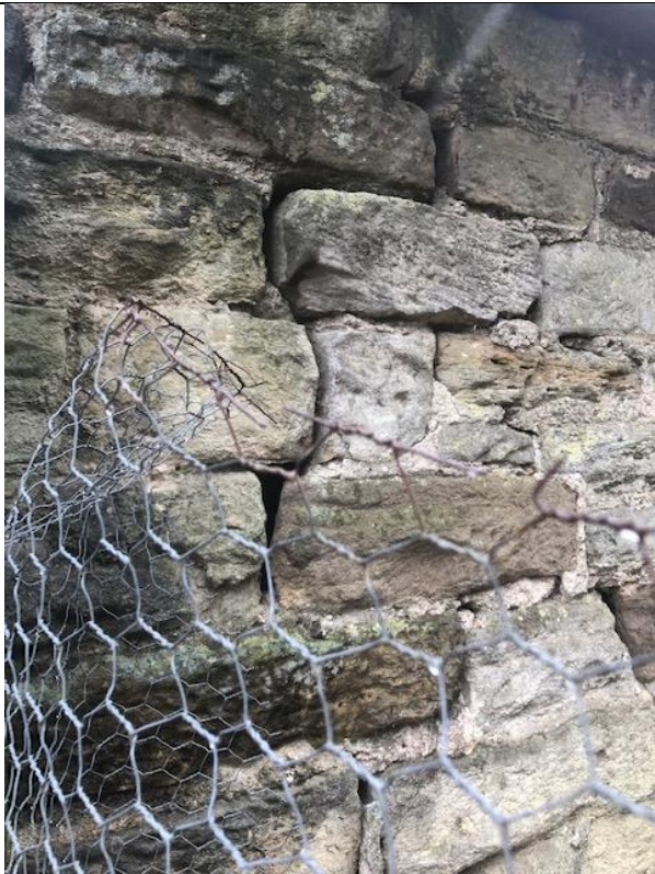
Photograph 7. Showing the damage on the other corner and north eastern elevation, leading into a large void behind.
