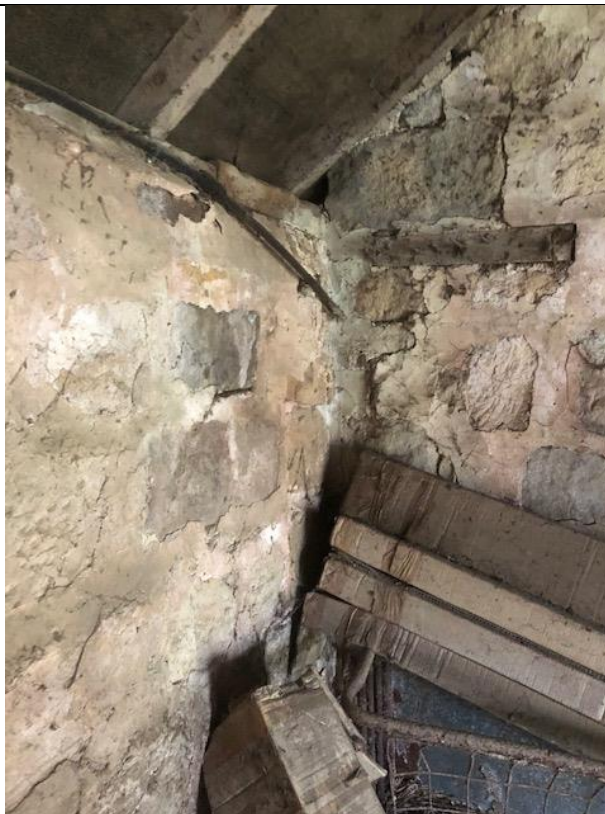
Photograph 29. Showing the voids in the corner of the room.
