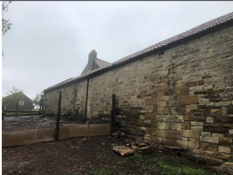
Photograph 10. Showing the other side of the north eastern elevation with the blocked up door and the hole with the deep void visible centre right edge of the picture.
