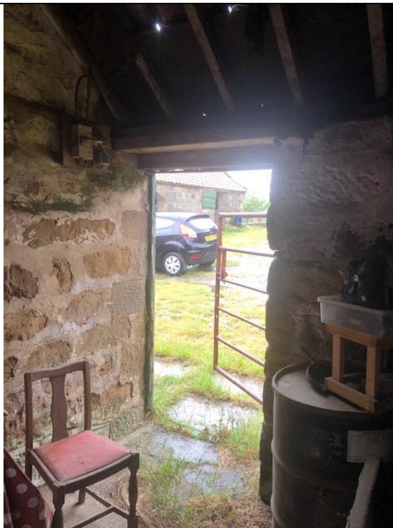
Photograph 27. Showing the doorway of the storage room/ office, with the gap in the corner of the wooden lintel and damage to the roof.
