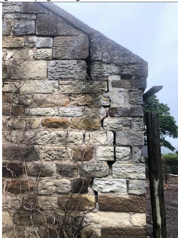
Photograph 6. Showing the coping damage on the south eastern elevation, right hand side with the large running split in the pointing and stone work.
