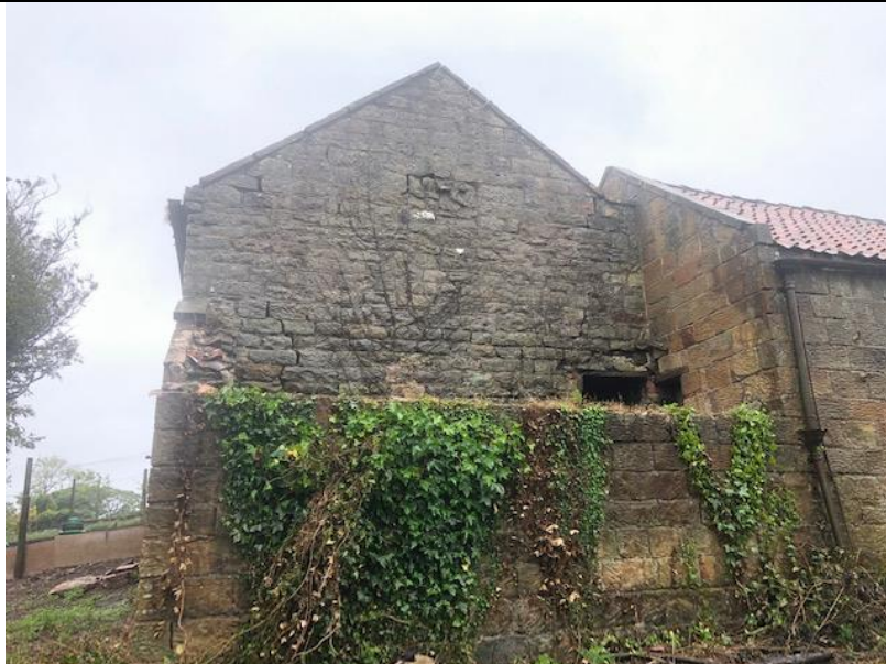
Photograph 11. Showing the north western elevation with the lean too that has been partly demolished. Note the damage to the stone work and pointing at high levels.
