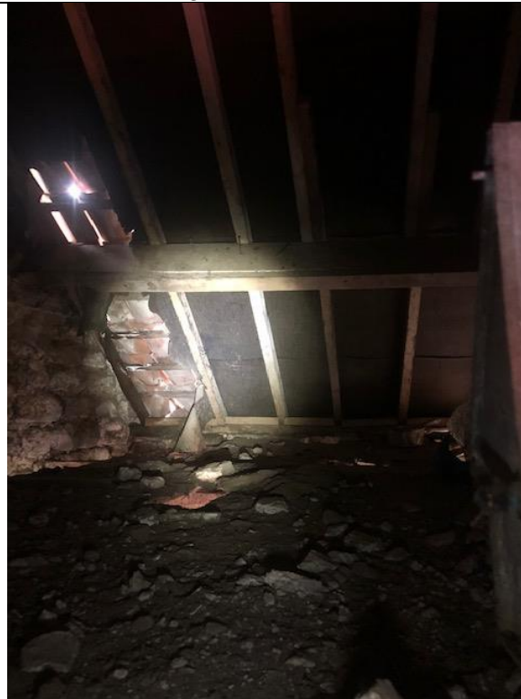
Photograph 24. Showing the first floor room with lots of debris and damage to the roof (daylight visible). Floor boards are rotten, door access from the adjacent room.
