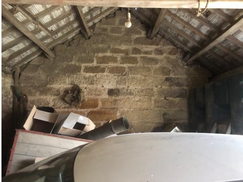
Photograph 18. Showing the gable end of the storage area (which joins to the stables) with the timber framework and wooden backing to the tiles. Gaps present where the timbers join the wall and in each corner of the bottom of the apex.
