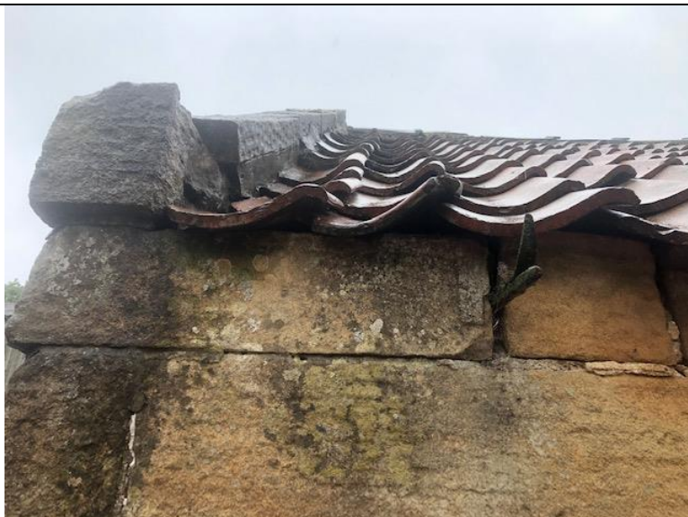
Photograph 9. Showing the tiles on the north eastern elevation with gaps under the tiles present.
