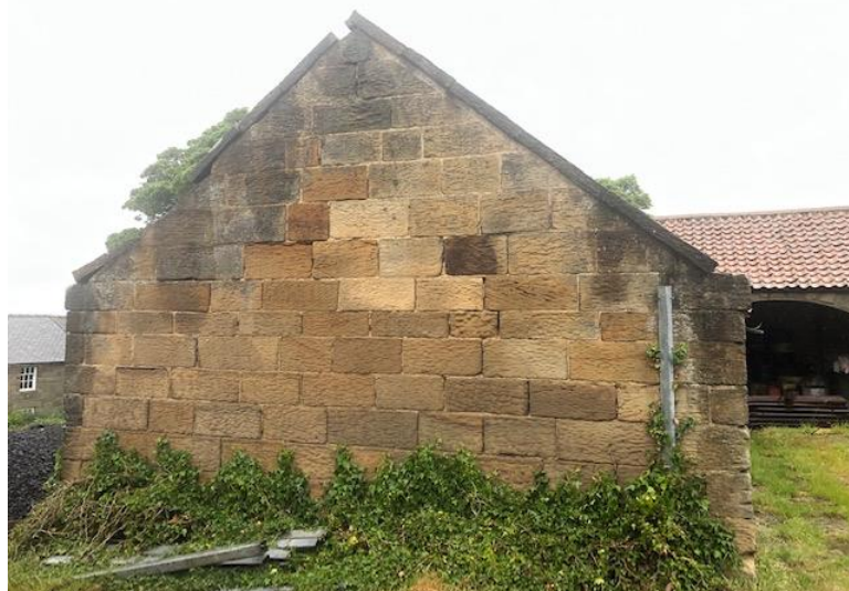
Photograph 14. Showing the gable end of the south western elevation with other side of the damage to the coping stones with shallow erosion to the stone work and ivy creeping up (possibly cut back at an earlier point in time).
