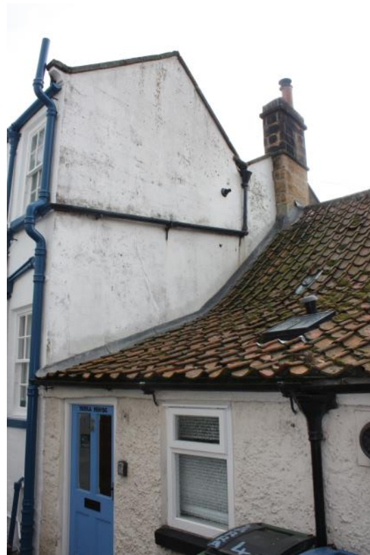
Photo 5: View of west gable of No. 5 Bloomswell, with north elevation of No. 4 Bloomswell (Yarra House) in the foreground
