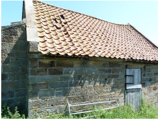
Photo 1 Barn 1 showing missing tiles
