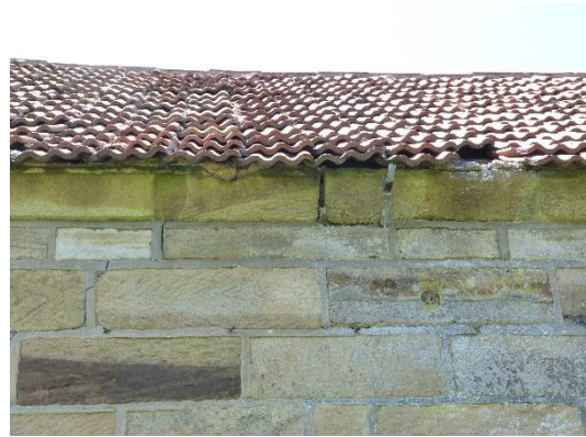
Photo 10 Gaps at eaves in Barn 2
