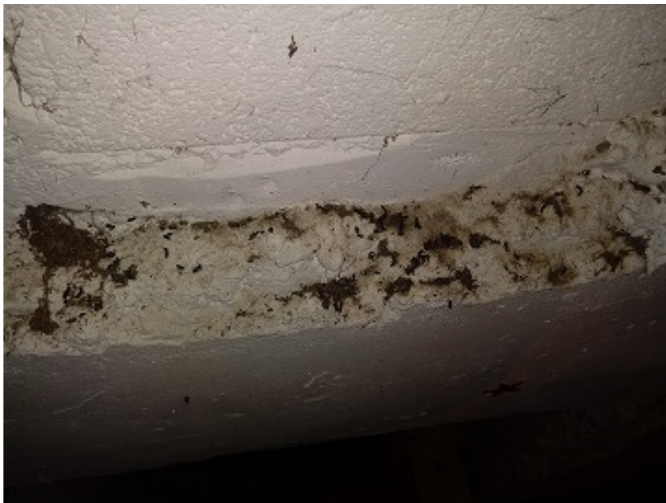
Plate 6. Shows evidence of bat habitation in form of bat droppings on south gable wall ledge.
