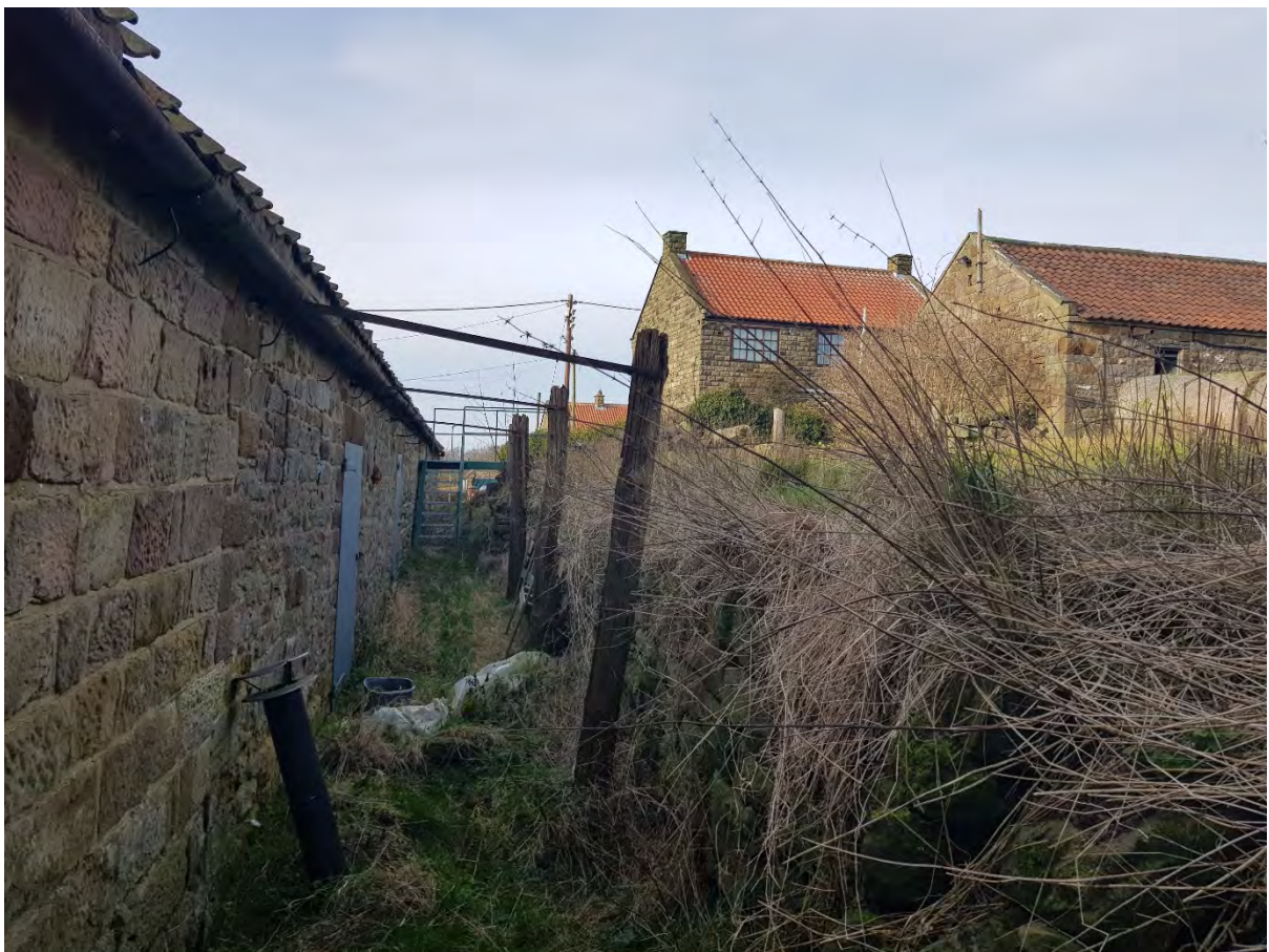
6. View of rear of outbuilding looking west (steel stairs proposed to be removed)
