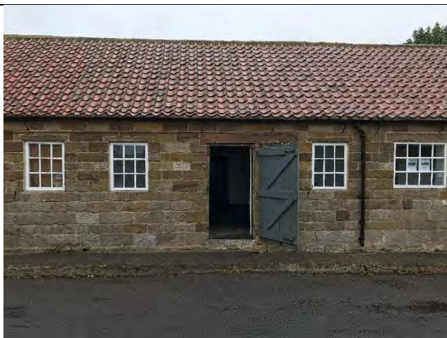
Typical Unit front with Ledge & Brace door and Georgian style softwood windows.
