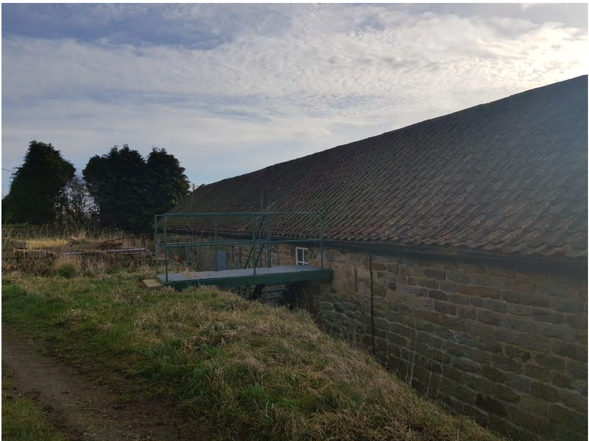
4. View of rear of outbuilding looking east from track (steel stairs proposed for removal).
