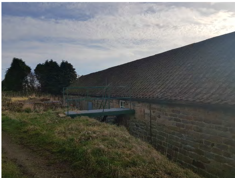
5.28 View of steel stairs fire escape at rear of building: Proposed to be removed.
