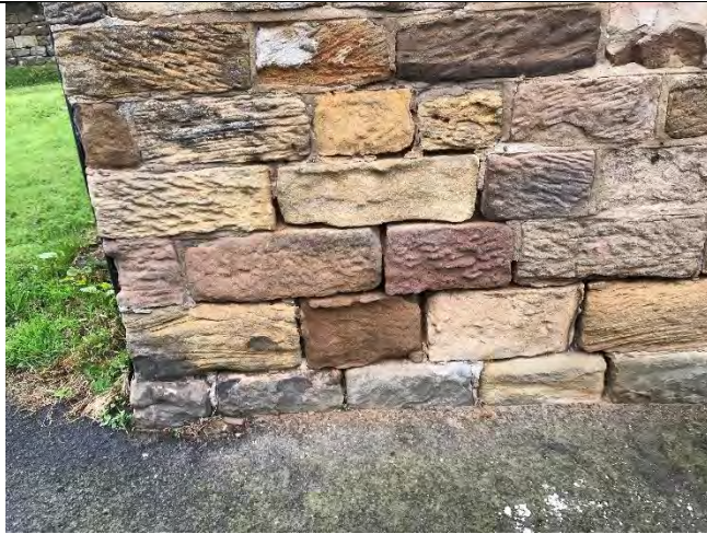
South Elevation- Lime mortar pointing required
