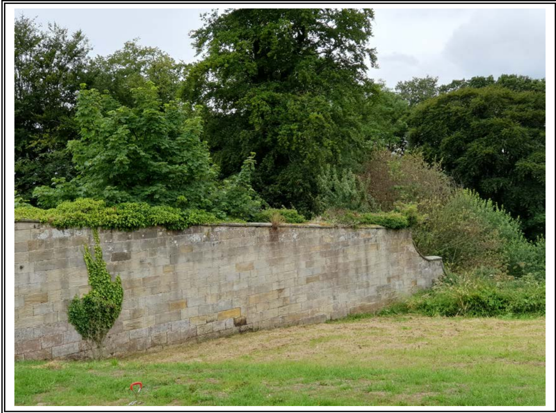
Photo 7 North side of garden wall. Shed to be built on the other side of this wall.
