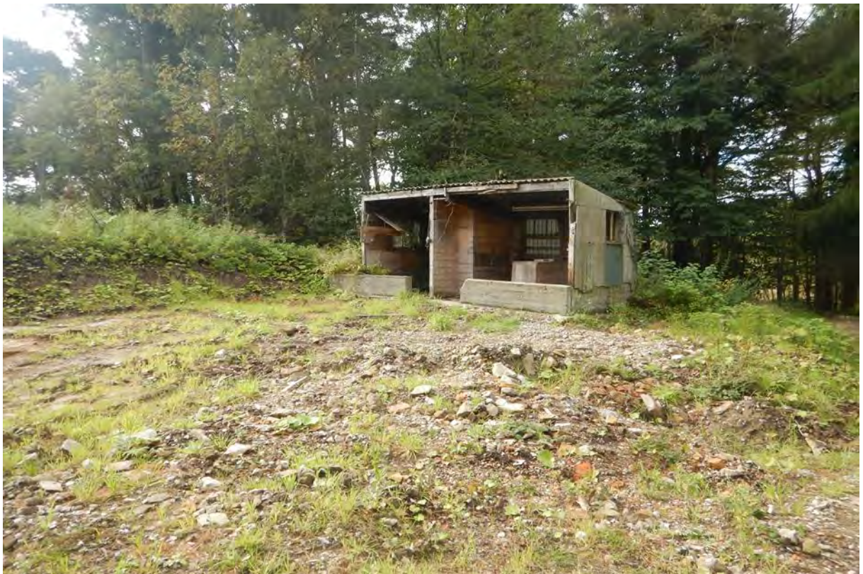
Plate 2. Derelict Building in SW corner of the Proposed Development Area.
