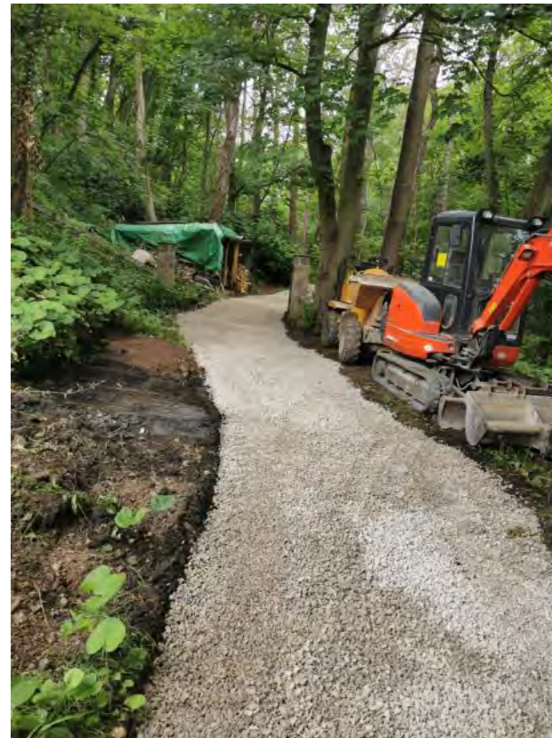
Typical new track construction. The photos show examples of how typical tracks will look immediately upon completion. Note that the areas alongside the track is constructed of banked earth and will be colonised with native undergrowth over the subsequent growing season.
