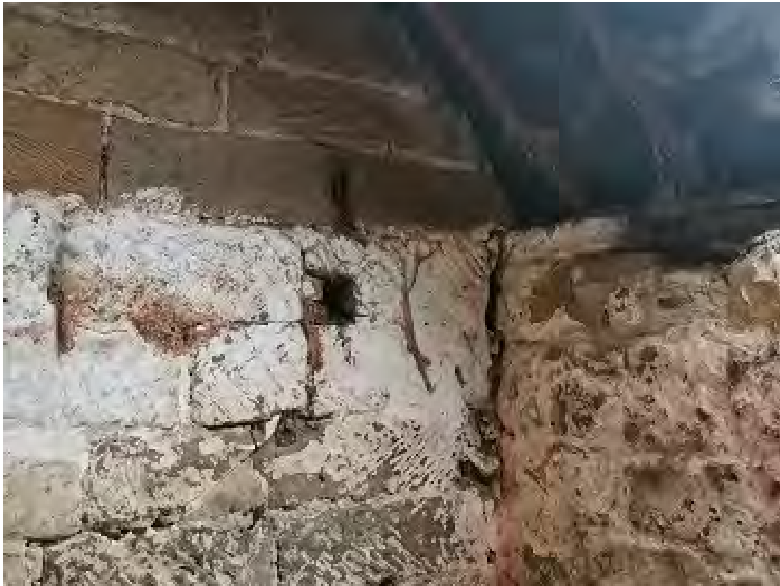
Plate 2 Example of holes in internal walls
