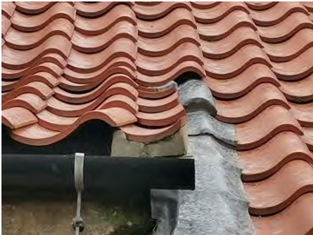
Plate 9. Shows lifted pantile and bird spikes under header tiles on the western elevation.
