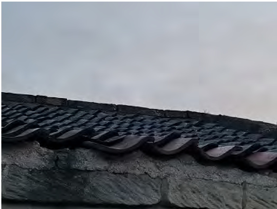
Plate 6. Shows lifted pantiles
