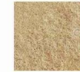
Existing paint layers to the existing natural stone detailing to fenestration to be removed
