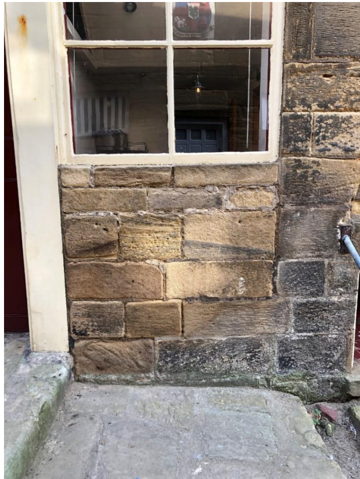
Photograph 1 Vertical joint in the stone work
