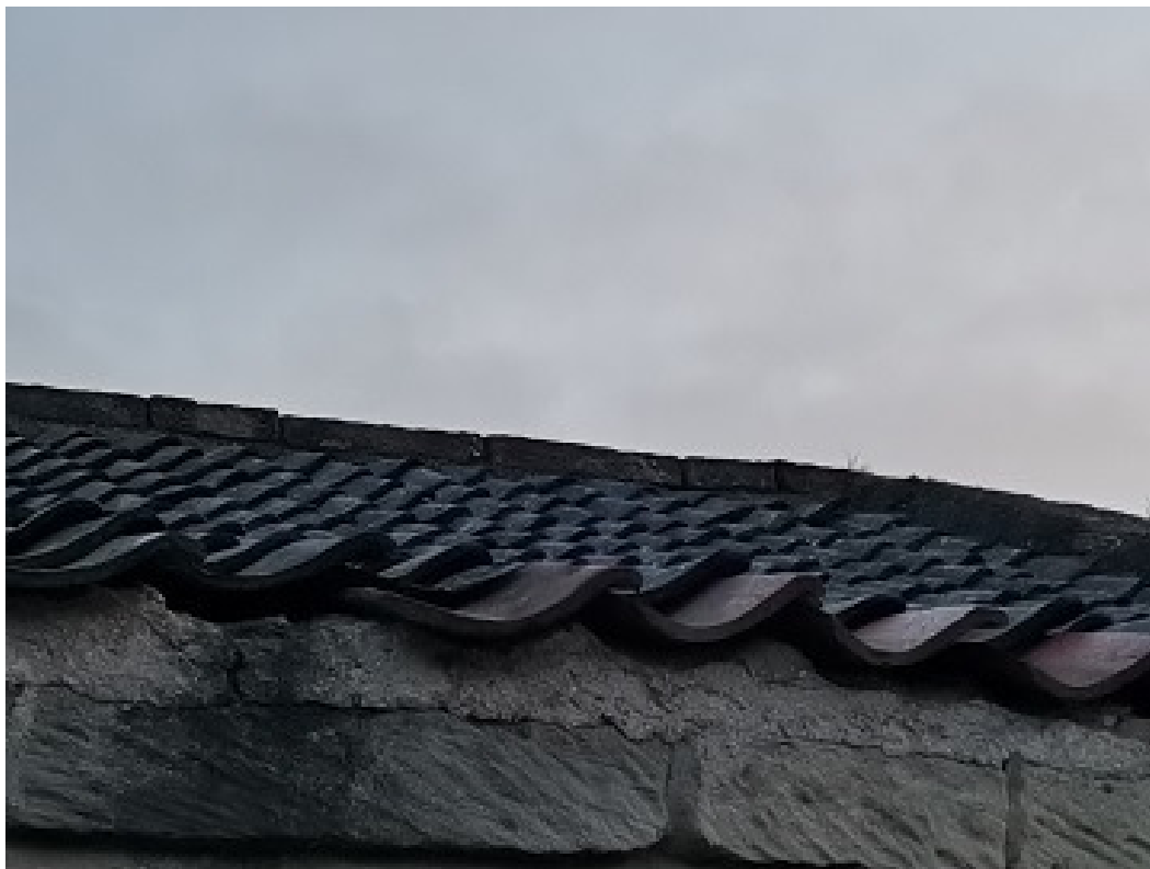
Plate 6. Shows lifted pantiles
