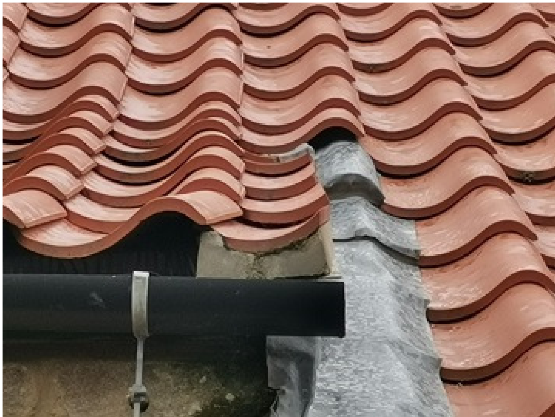
Plate 9. Shows lifted pantile and bird spikes under header tiles on the western elevation.
