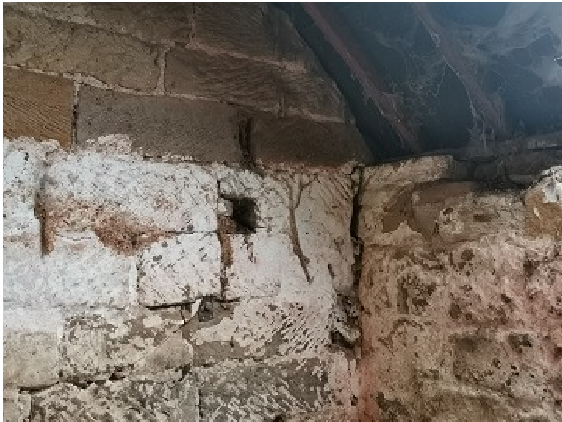
Plate 2 Example of holes in internal walls
