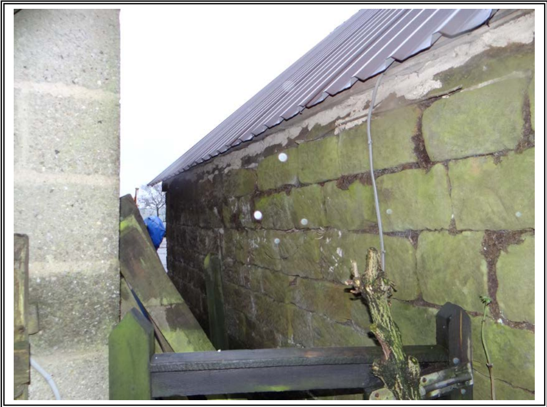
Photo 2 Rear (north) elevation. Section needs reconstructing.
