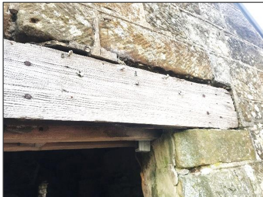
Photo 6. Crevices around lintel.
