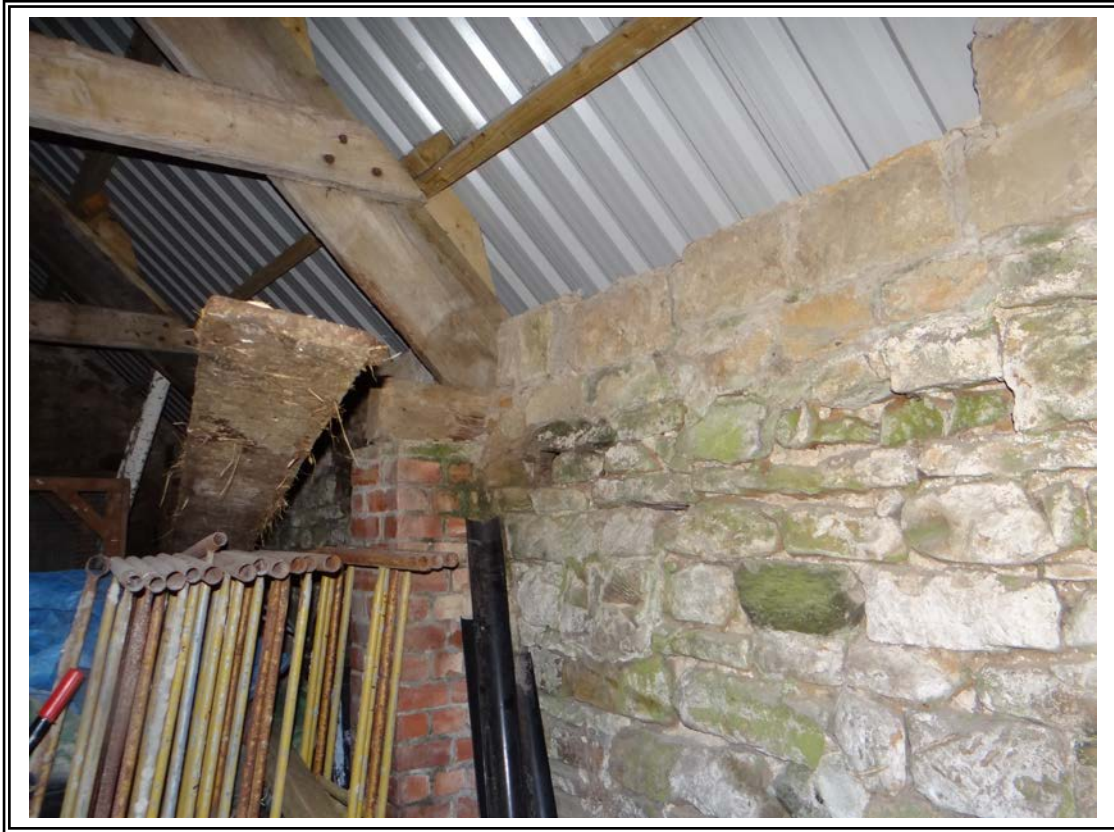
Photo 5 Inside face of the rear wall and underside of the roof covering.
