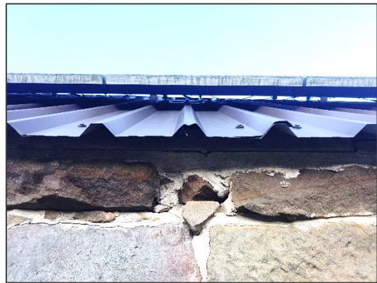
Photo 5. Large gap between solar panels and roof.
