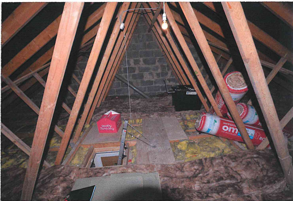
Photograph of the existing roof space which is generous and has head space of about 2.7m.
