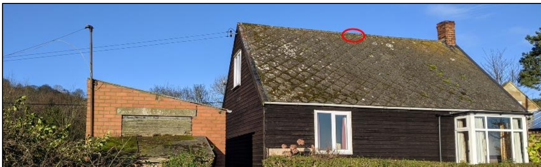
Plate 1. Southeast elevation of B1 (main dwelling), with B2 (brick outbuilding) on left. The identified bat roost location is circled in red
