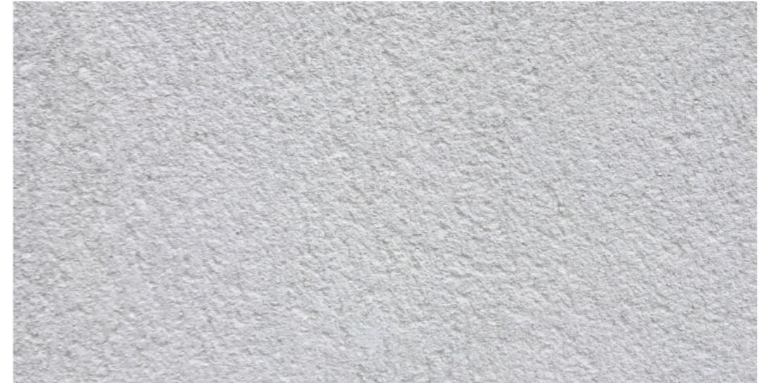
Crestbank - Existing render detail photograph
