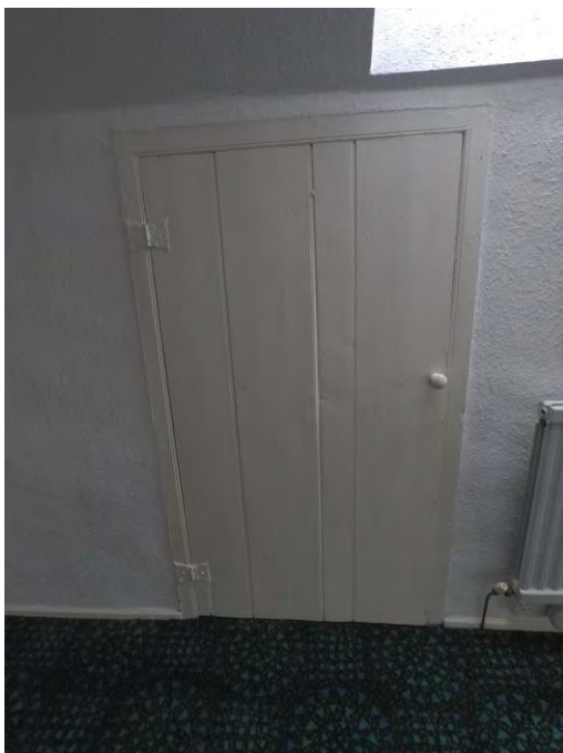
Photo 47: Cupboard door & paneling
