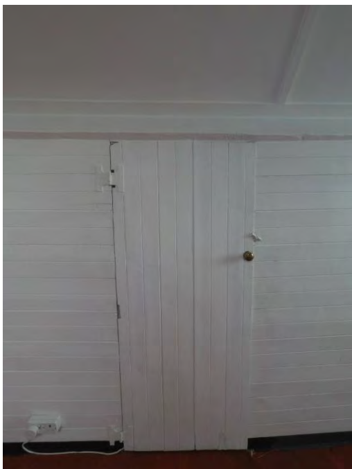
Photo 43 Cupboard door & paneling
