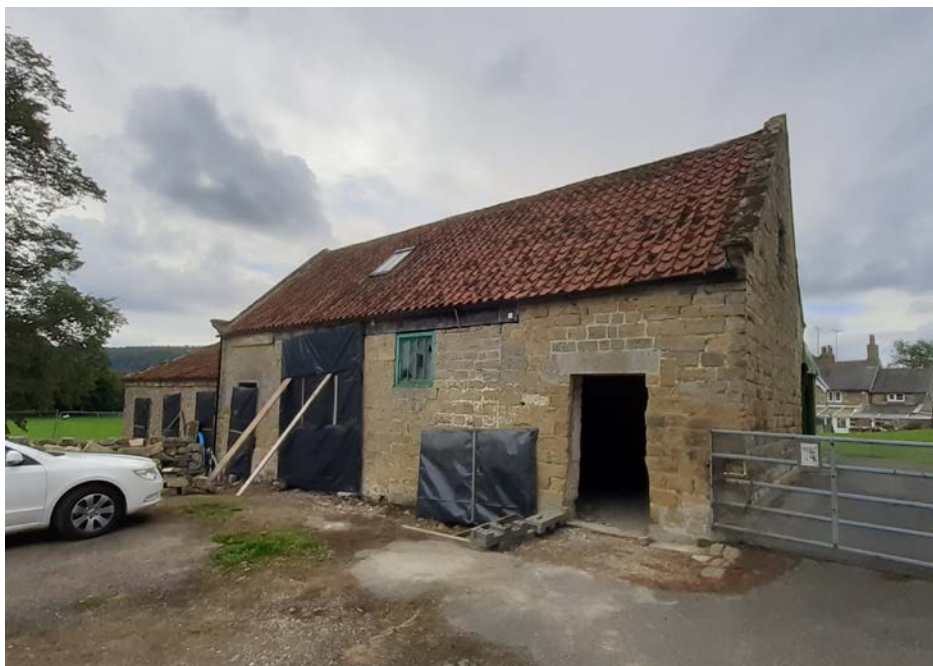
Front elevation of barn showing existing blocked up cart door opening to be re-opened
