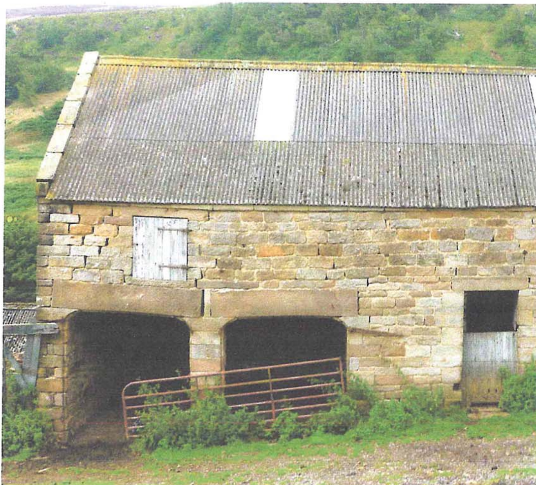
Photo 1 Photo of front (west) elevation of building A (barn) showing settlement of pier and dropped masonry over
