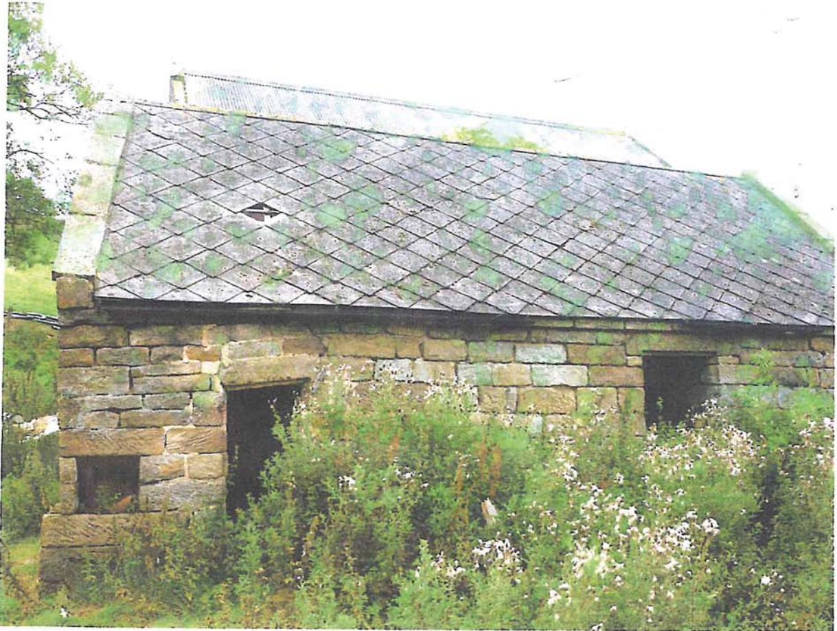
Photo 2 Photo of east elevation of building B showing settlement of south east corner of masonry
