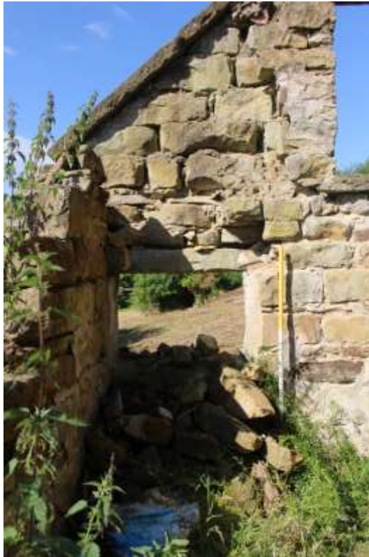
Plate 53: internal view WSW of pigsties W partition showing blocked doorway— Building No. 1
