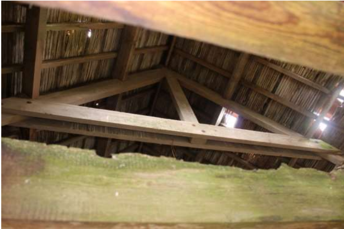
Plate 133: Internal view ESE of king post roof truss within the first compartment of Building No.4
