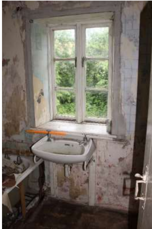
Plate 75: Internal view NNW of 1 st floor bathroom showing two light casement window within N wall – Building No.1
