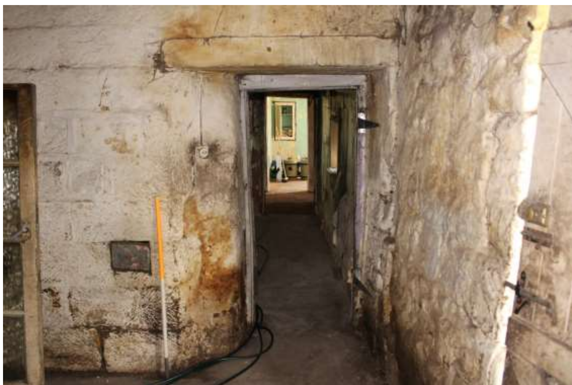
Plate 50: internal view NW within ground floor outhouse showing entrance from kitchen and soot box – Building No. 1
