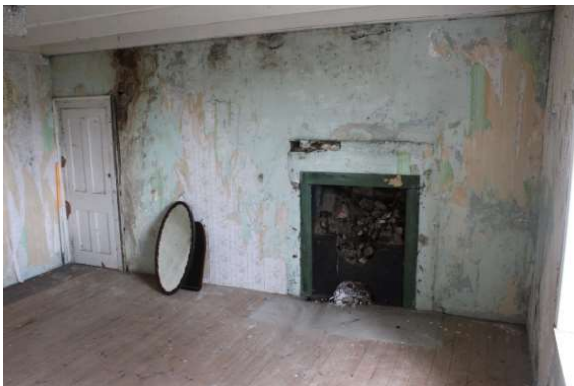
Plate 82: Internal view NE of 1 st floor fourth bedroom showing fireplace and locked storage alcove– Building No.1
