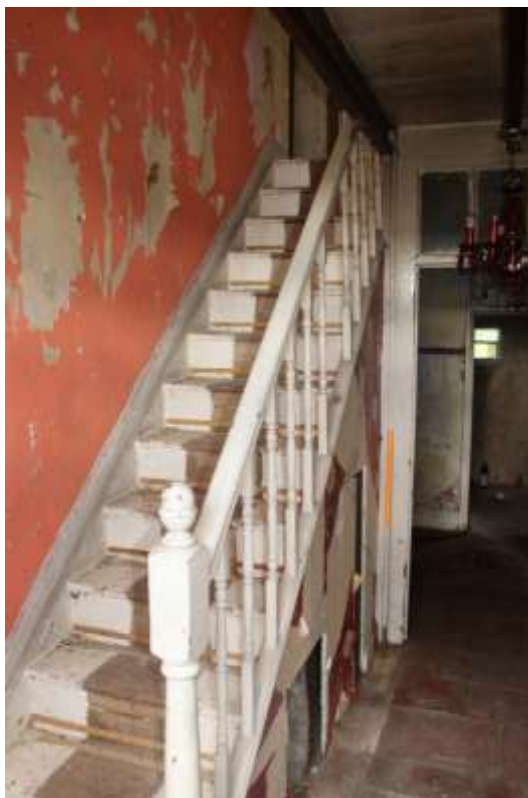
Plate 14: Internal view NW showing ground floor staircase within the farmhouse – Building No. 1
