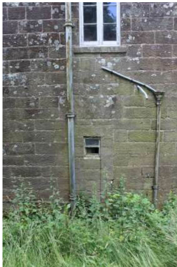
Plate 10: View SSE showing blocked central door within N facing elevation of the farmhouse (Building No. 1)
