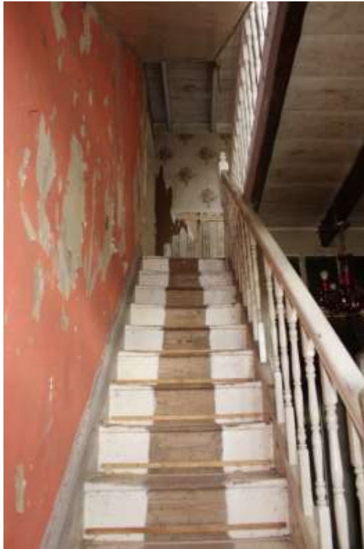
Plate 15: Internal view NNW showing ground floor staircase within the farmhouse – Building No. 1
