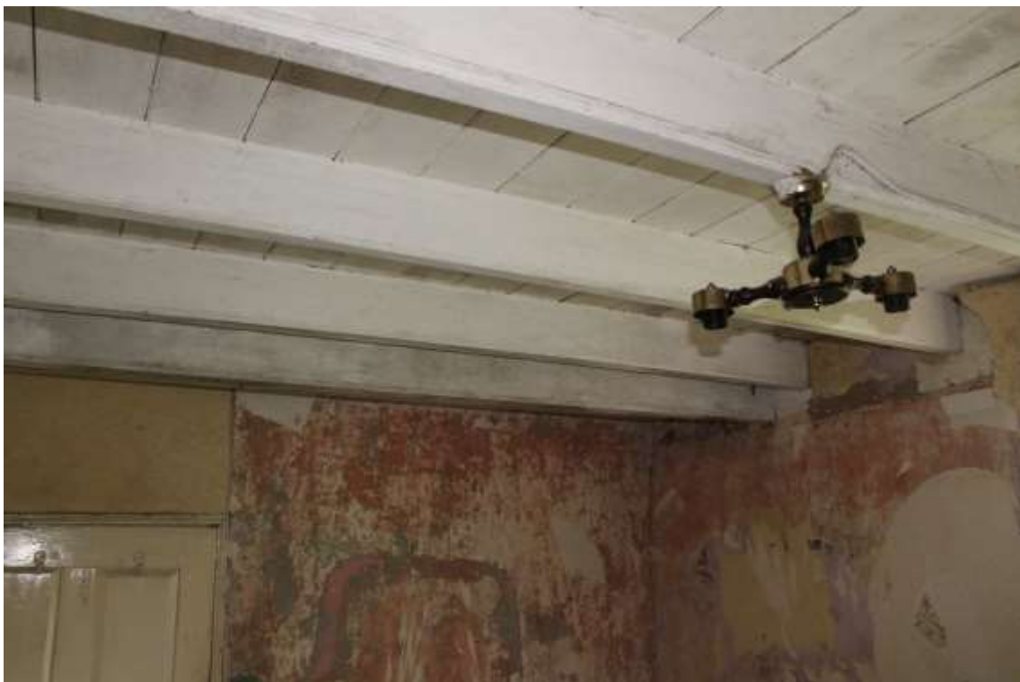
Plate 80: Internal view WNW of 1 st floor third bedroom showing ceiling – Building No.1
