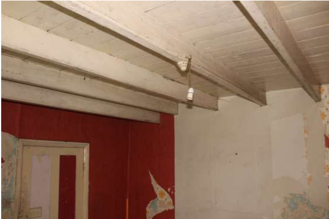
Plate 73: Internal view SE of 1 st floor second bedroom showing ceiling – Building No.1
