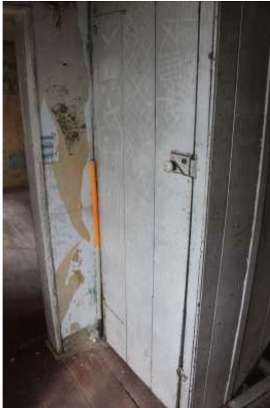
Plate 63: Internal view NW of 1 st floor central hall way showing attic stairs entrance— Building No.1
