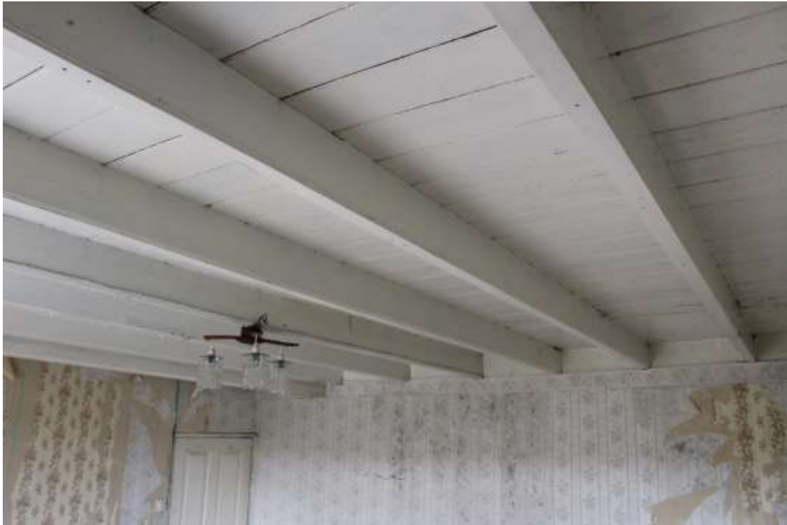
Plate 85: Internal view WSW of 1 st floor fourth bedroom showing ceiling – Building No.1
