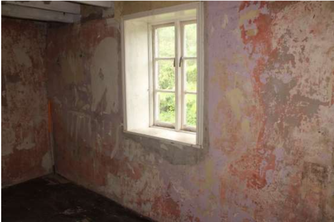
Plate 79: Internal view NW of 1 st floor third bedroom showing two light casement window with N wall – Building No.1
