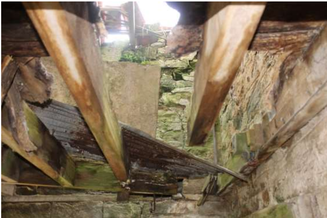
Plate 132: Internal view S of rotten ceiling timbers within the first compartment of Building No.4
