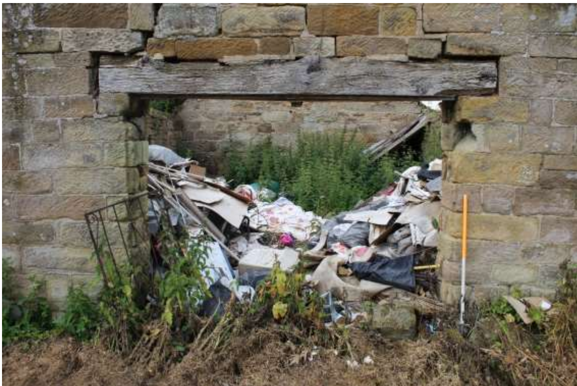
Plate 100: Exterior close up view E elevations of Building No. 2 and internal area
