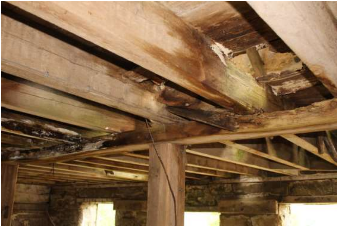
Plate 131: Internal view ESE of rotten ceiling timbers within the first compartment of Building No.4
