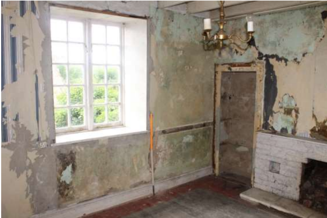
Plate 23: internal view SW within ground floor living room showing casement window within S wall— Building No. 1
