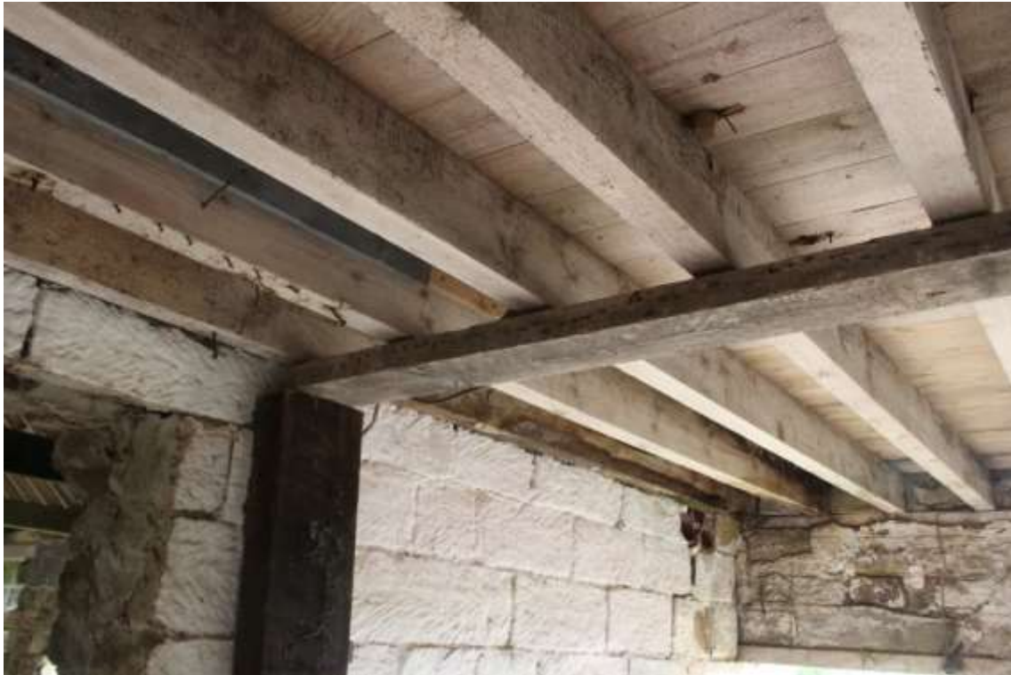
Plate 141: Internal view SSE of the roof timbers within the second compartment of Building No.4
