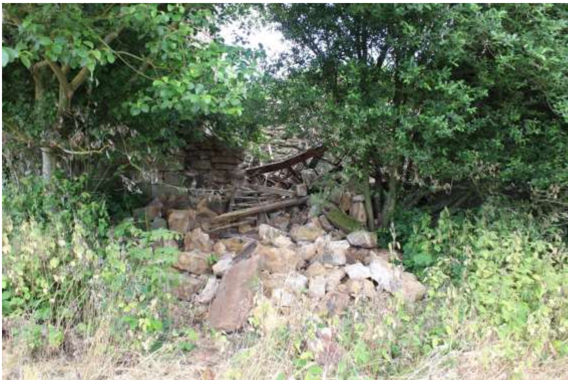
Plate 122: External views N of the collapsed third section of the S-facing principal elevation
