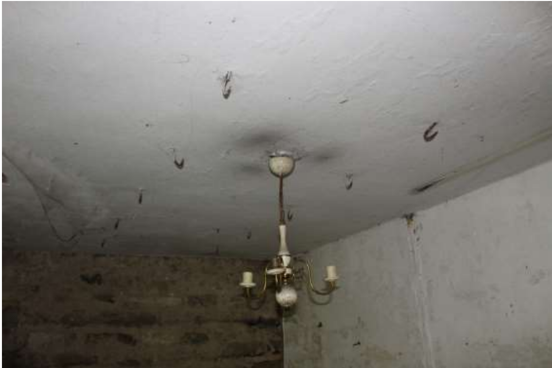
Plate 37: internal view E within ground floor storage room showing ceiling hooks – Building No. 1
