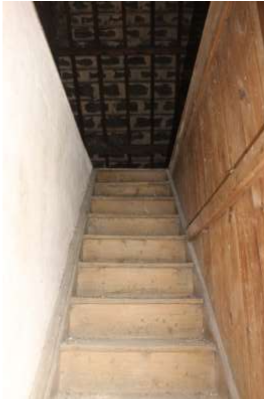
Plate 87: Internal view NNW of stair case leading to attic/roof space – Building No.1
