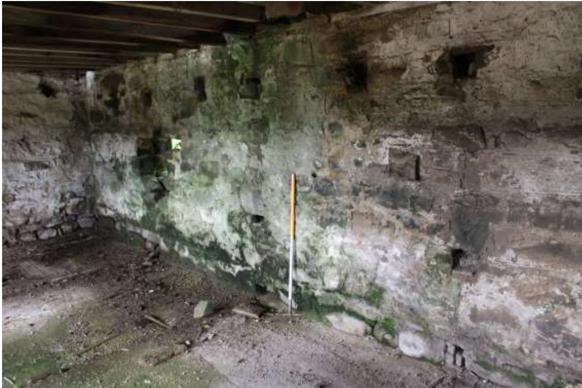
Plate 135: Internal view NW showing fixtures on the N wall aligned with the struts within the first compartment of Building No.4
